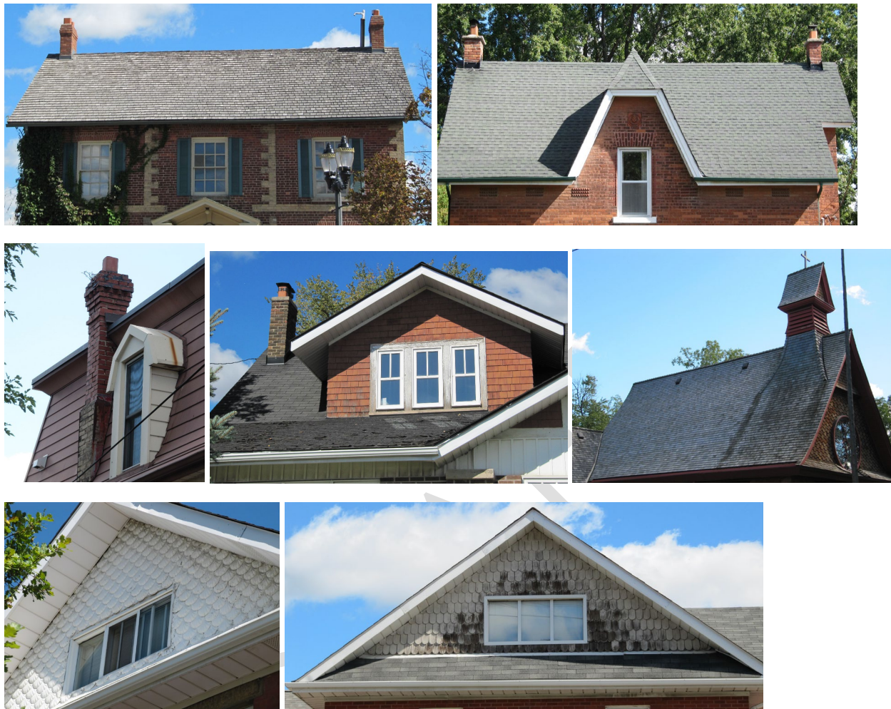
Photo 4.1: Examples of roof materials, shapes, pitches, and other elements in the HCD (chimneys, dormers, cupola)
