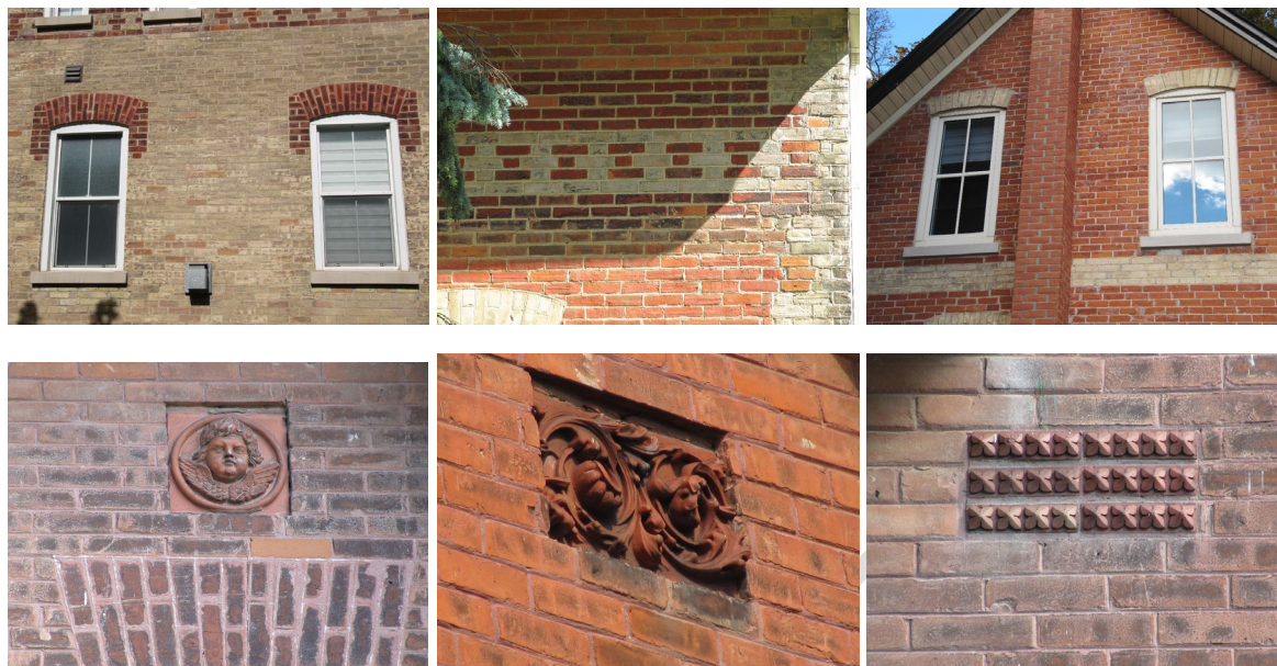
Photo 4.2: Examples in Core Maple HCD of red and buff brickwork and brick detailing including voussoirs, drip moulds, horizontal banding, quoins, and decorative clay elements in brickwork
