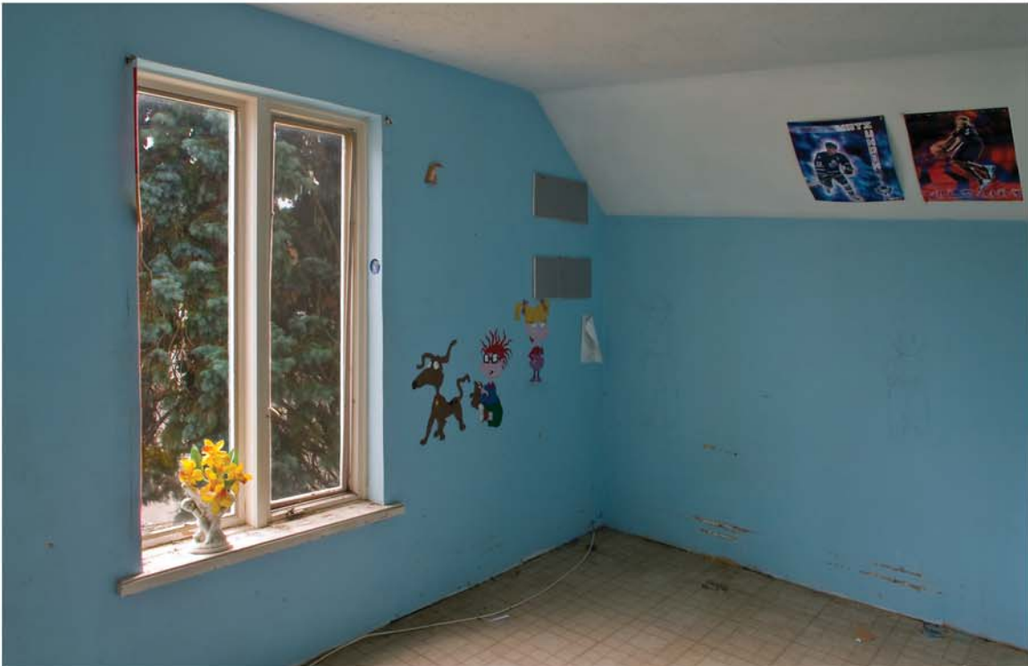
South West Bedroom, Looking South West, Showing New Enlarged Window On The South Elevation, No Window Trim Or Baseboard
