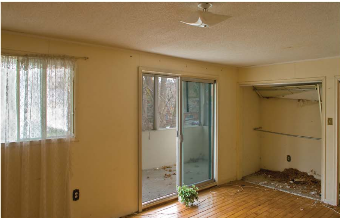
Master Bedroom Looking South East Showing New Sliding Doors To Enclosed Deck On The East Elevation
