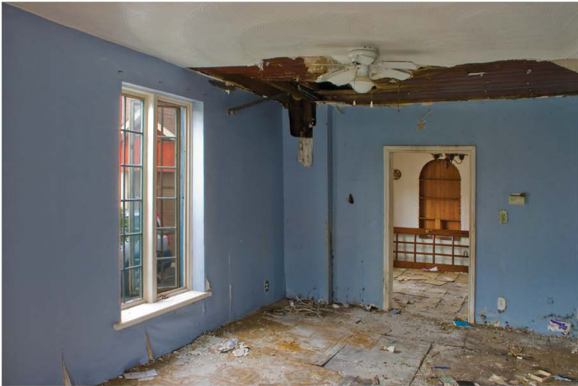
Living Room Looking North - East: Showing Replaced Window, Original Stained Wood T & G Ceiling with Drywall Over, Step Down Entry Doorway To Dining Area, And No Original Trim
