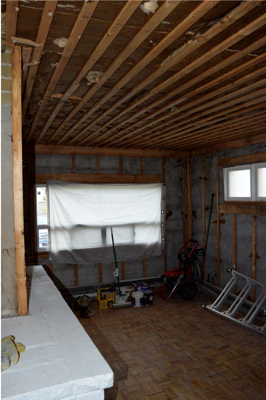
Image 18: Interior of addition, interior of brick walls have been parged, facing west
