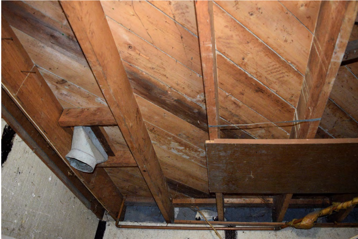
Image 24: Typical floor joists and subfloor construction, joists are 2" x 6" set 16" on center
