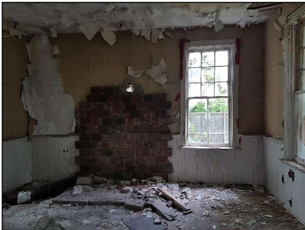
Figure 60: Looking north within the first floor of the existing building towards the north elevation
