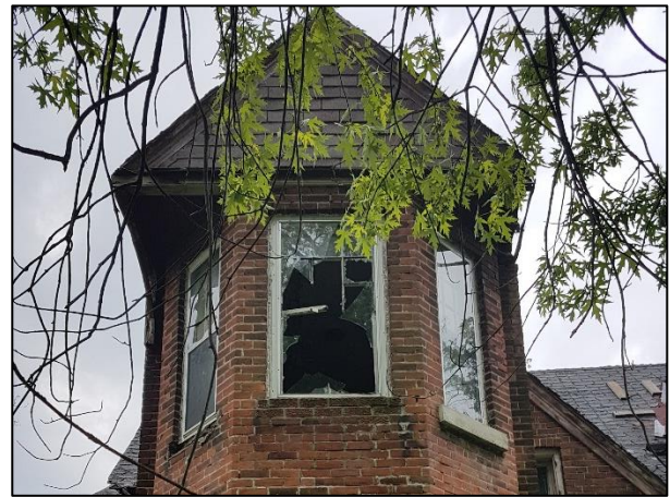
Figure 33: East elevation detail showing window openings and broken windows at the second storey (ASI 2019)
