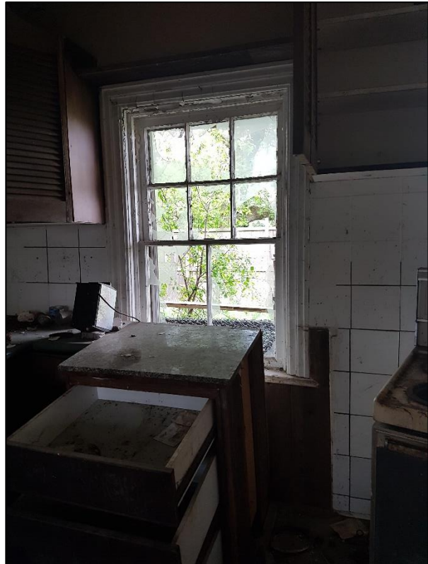
Figure 55: Looking south within the kitchen at the west end of the building, showing the existing window (ASI 2019)
