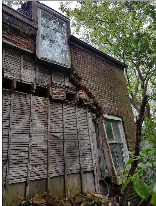
Figure 47: North elevation detail showing deteriorated and missing exterior wall, dormer window and first-floor window opening (ASI 2019)
