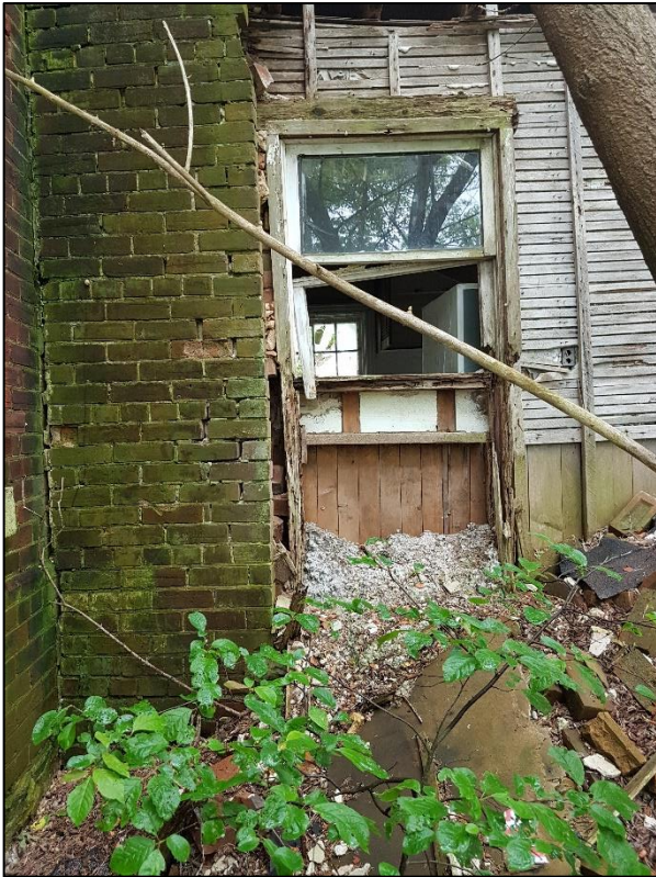
Figure 46: North elevation detail showing deteriorated exterior wall and first-floor window opening (ASI 2019)
