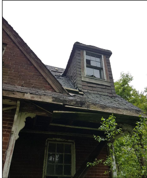
Figure 41: East elevation detail showing the deteriorated porch roof and dormer above the porch
