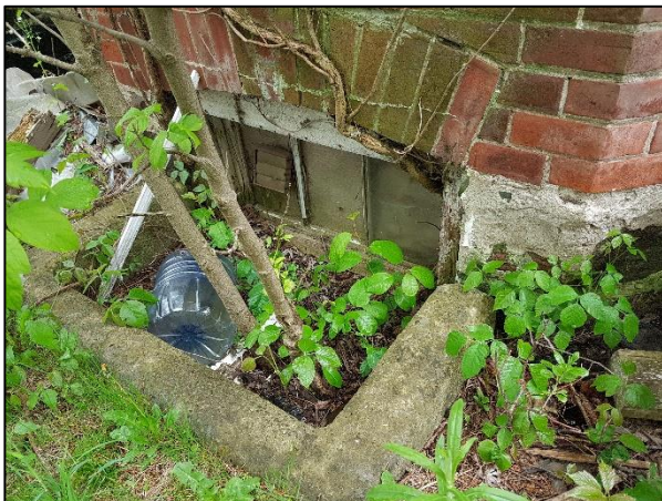
Figure 34: East elevation detail showing segmentally arched basement window openings and parged foundation (ASI 2019)
