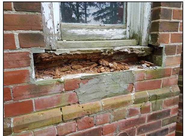
Figure 35: East elevation detail showing missing sill and deteriorated window (ASI 2019)
