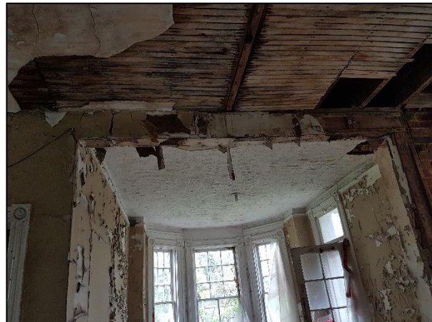
Figure 61: Deteriorated first-floor ceiling within the east end of the existing building
