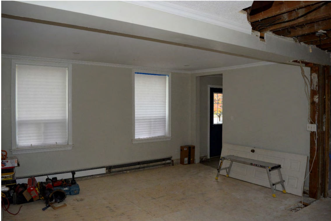
Image 14: First floor interior, note bulkhead indicating original location of internal wall, facing northwest
