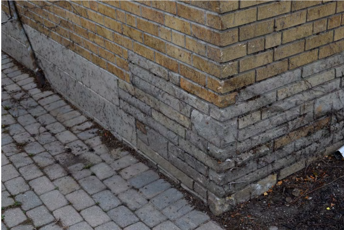
Image 11: Cement block foundation of north addition with decorative ashlar cement block used on front facade
