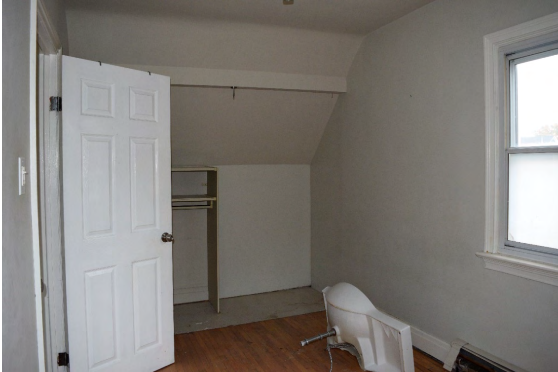
Image 20: North side bedroom, note original flooring and modern hollow core door, facing west
