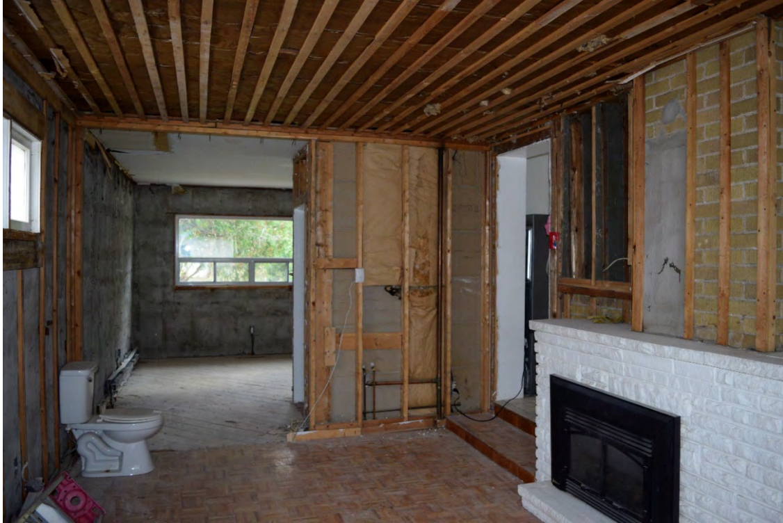
Image 16: Interior of north addition, fireplace is contemporaneous to the addition, facing east
