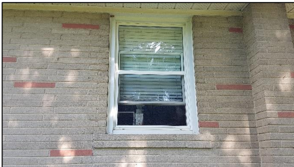
Figure 16: Window on the east elevation with brick sills that are found throughout the house (ASI 2019)
