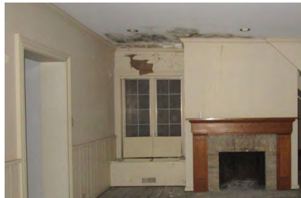
Ground floor interior depicting mould and water damage on wall and ceiling (ERA, 2019).
