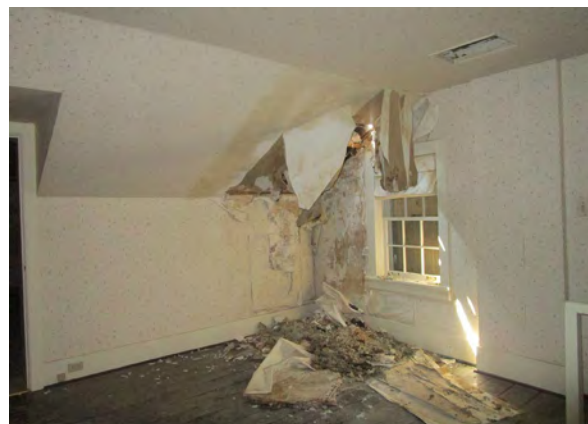
Second floor interior depicting defective roofing area (ERA, 2019).
