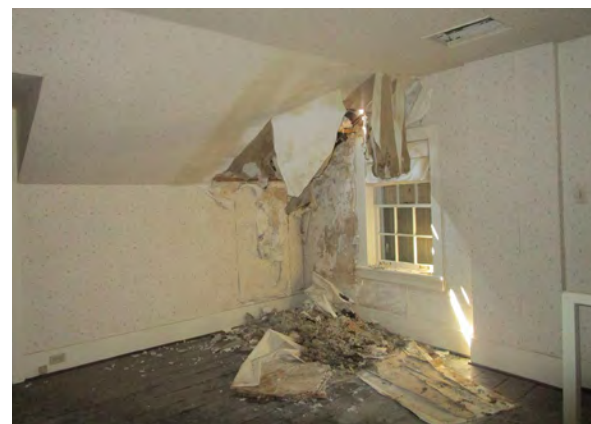
32. Evidence of defective roofing in southwest corner of the house (ERA, 2019).
