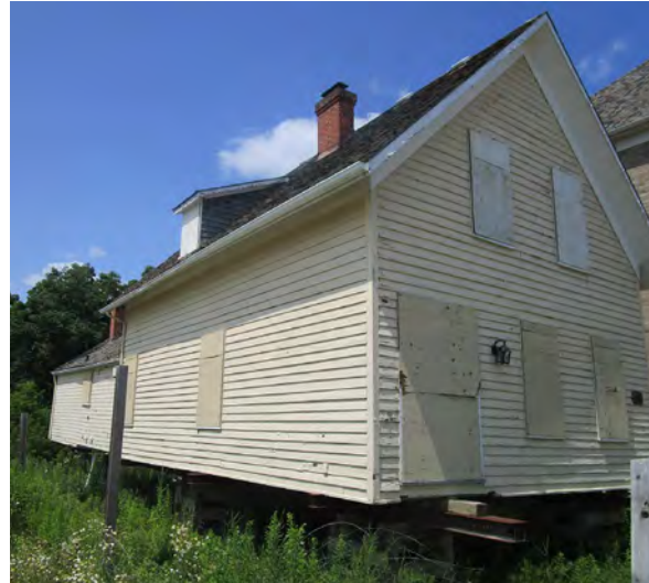
5. Current condition of the George Munshaw House (ERA, 2019).
