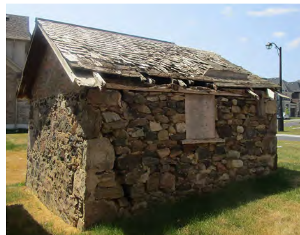
33. Smokehouse structure requires rebuilding and repointing of walls(ERA, 2019).
