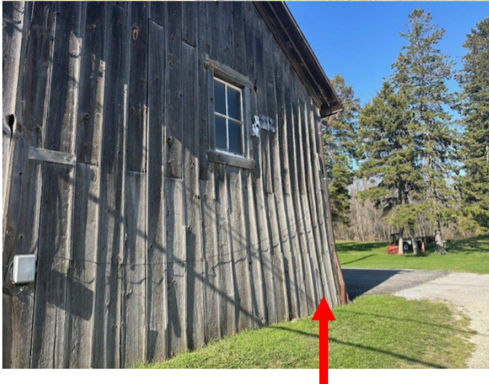
Structural damages on the southeast side of the barn
