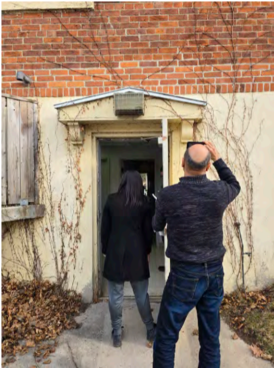
Detail of the current canopy above the basement door that was added in the 1980's.
