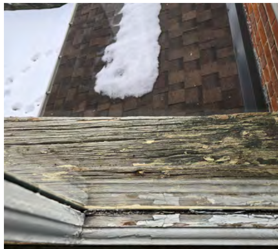
Detail of existing window sill of a window located on the east facade above the porch (second floor).
