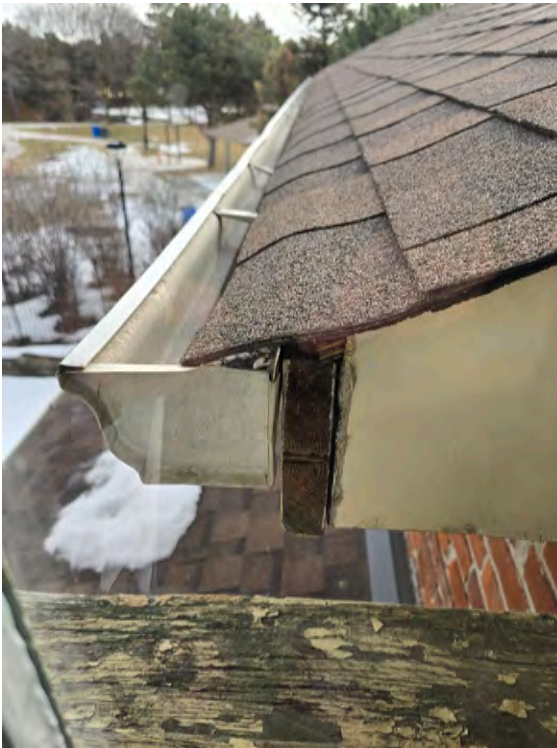
Detail of the current roof and eavestrough above the porch that was replaced.
