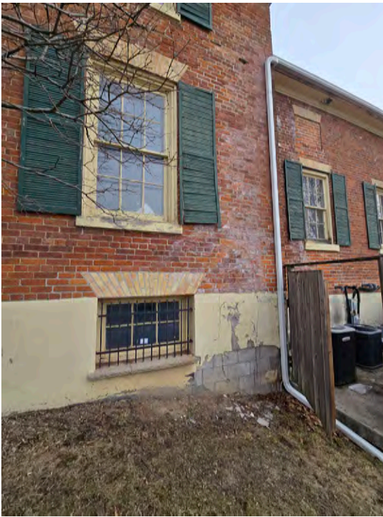
Detail of the current basement foundation that was built in the 1980's when the building was moved to its new location. The top of the photo illustrates the window opening filled in with masonry in the 1980's.
