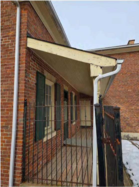
Detail of the shed above the porch that was rebuilt in the 1980's.
