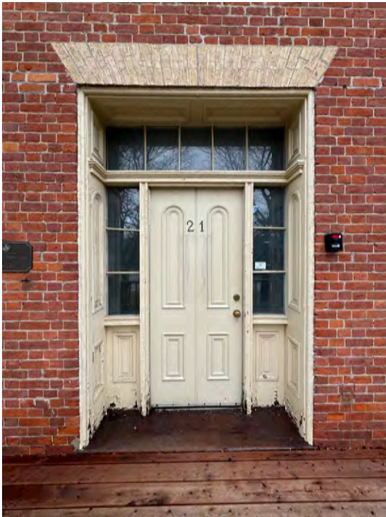
Detail of the original decorative wooden panelled reveal around the recessed front door.
