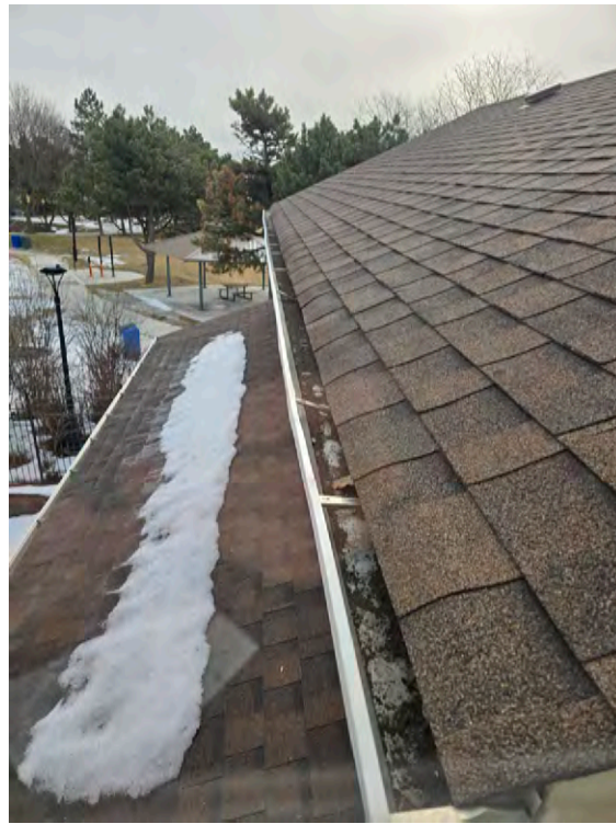
Detail of the current roof and eavestrough above the porch that were replaced in the 1980's. Asphalt shingle roofing was replaced recently.
