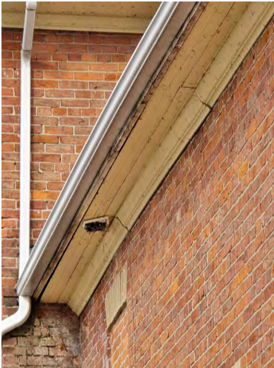
Detail of the current wood soffit and moulding, and eavesthrough and downspouts that were replaced in the 1980's.
