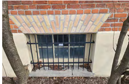
Detail of the lintel insert brick arches above the basement windows that was rebuilt in the 1980's. The welded security bars were added at the same period.
