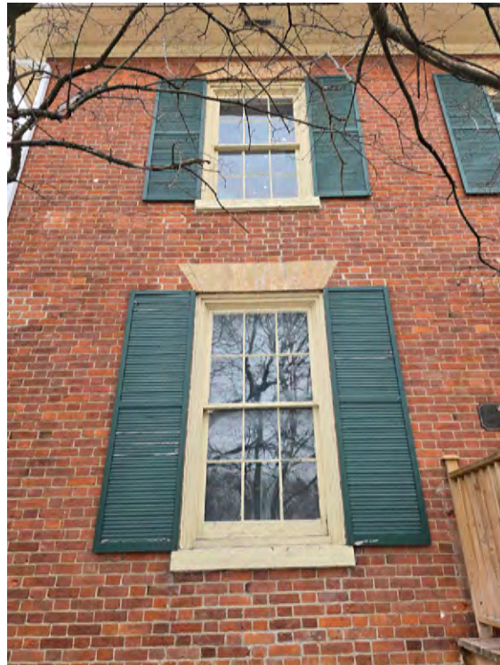
Detail of the current typical original windows where the wood window sills were replaced and the shutters were added in the 1980's.
