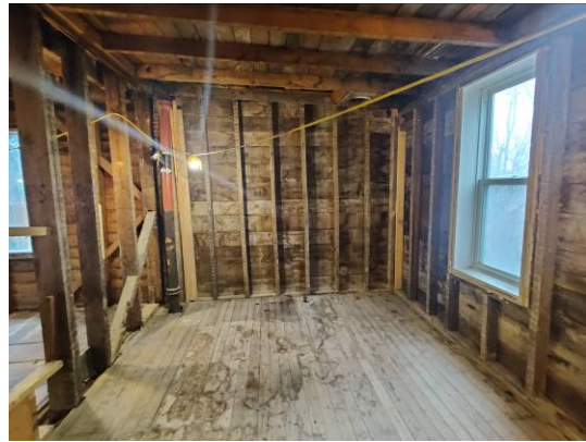
Figure 26. Kitchen tail, looking north. Note that walls are of sheathing, not clapboard. There may have been a different exterior finish. Board and batten was a common siding on kitchen tails.
