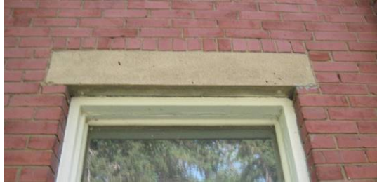
Figure 34. Lintels appear to be of homemade concrete castings rather than limestone or factory precast.
