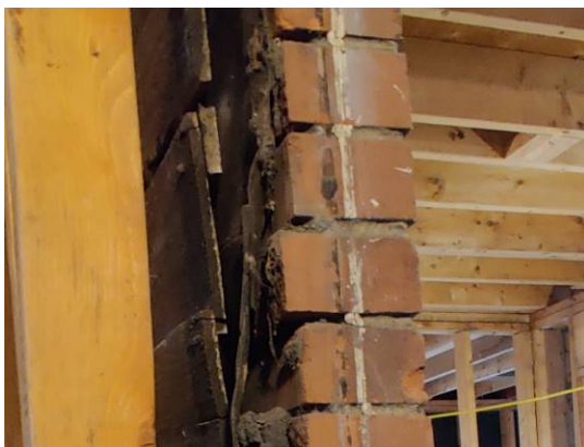
Figure 43. This was once an exterior wall: from left (inside) to right (outside)—stud, clapboard, roofing felt, air gap, brick. There might be some kind of ties between the brick but we haven't found any.
