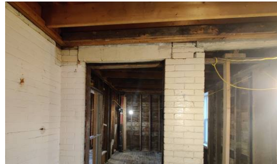
Figure 39. Settlement cracking at lintels on original ground floor kitchen tail.
