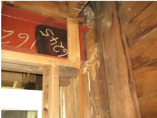
Figure 42. At some point a bearing wall on the ground floor was removed and replaced with a steel beam. It rests on a notch in the original framing and this timber salad. In my professional opinion, this is not proper bearing. My photo.
