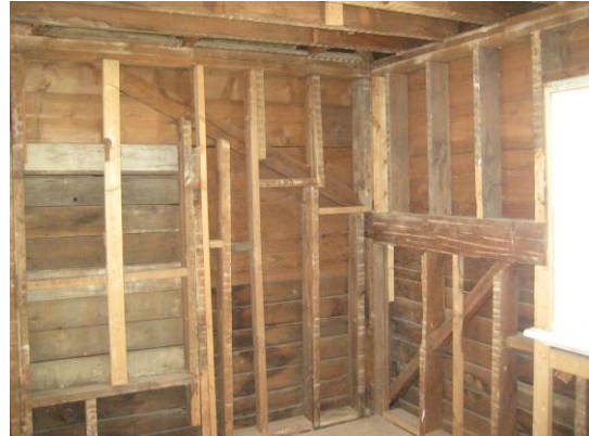
Figure 32. On the left, you can see filled-in original window in the south gable end. Note that its head is higher than the header beam to the right.
