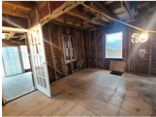
Figure 24. Northwest corner of the ground floor. The diagonally-braced corner post and door post are evident, as is the clapboard siding on both exterior walls.
