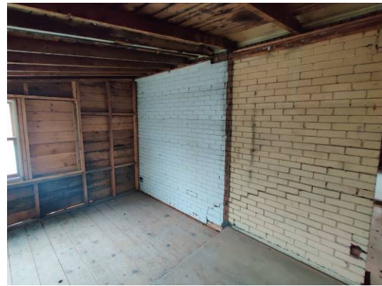
Figure 40. Settlement cracking, second floor rear wall.
