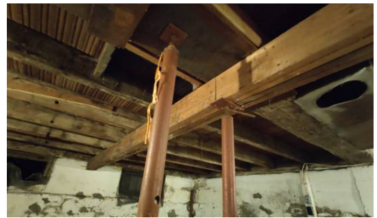
Figure 45. The ground floor framing, including the summer beam, has required some additional support. Unknown if this is related to the steel beam installed above. .
