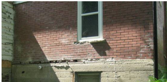
Figure 36. This sill on the rear wall has almost completely fallen apart. The bottom course of brick is crumbling, for reasons unknown, and the mortar has eroded in the lower right corner.
