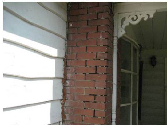
Figure 38. Mortar erosion on southwest corner of the house.
