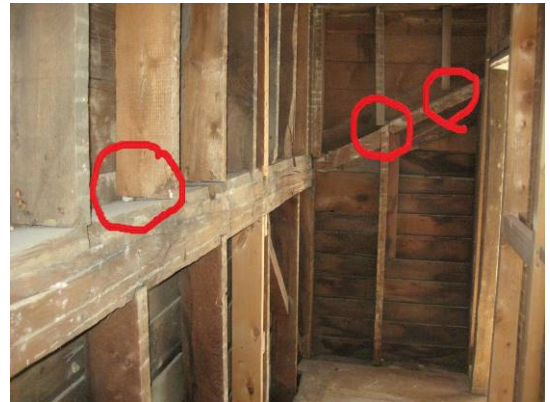
Figure 44. Some of the upper addition studs are not properly seated on the original top plate. My
