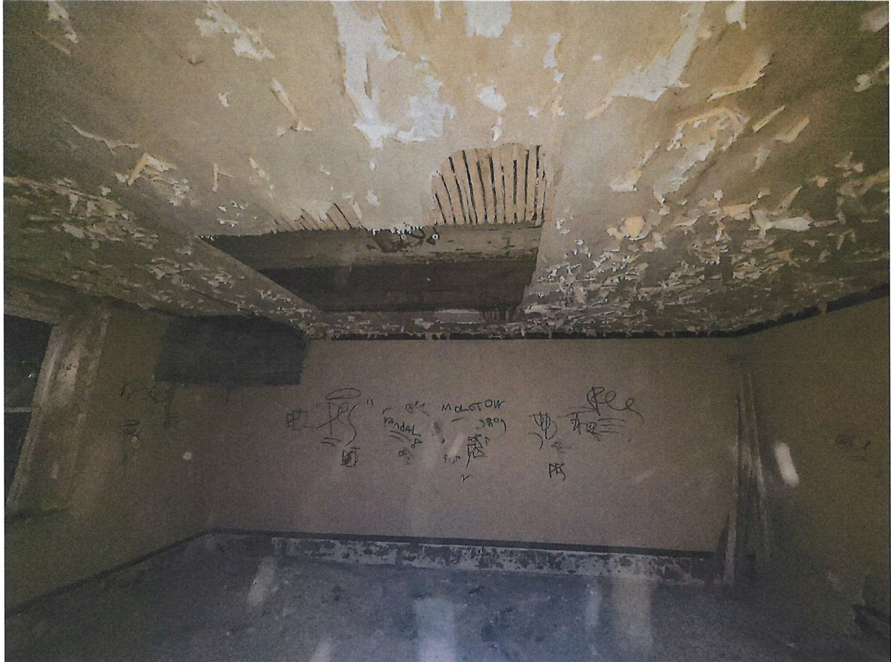
Photo 3 - Typical view of interior showing deteriorated finishes
