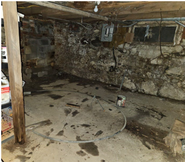
Figure 4: Water infiltration visible with discolouring of the slab due to water absorption throughout the basement.
