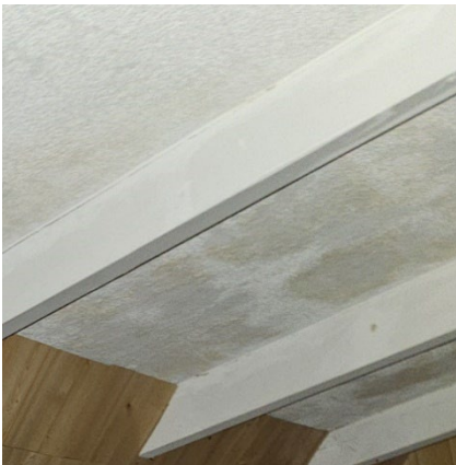
Figure 12: Ceiling mold and discolouration due to water penetration from roof.
