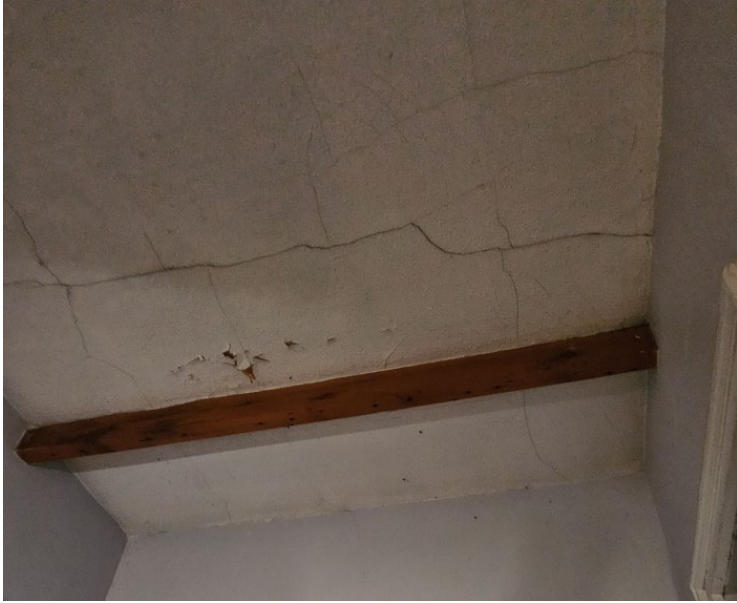
Figure 26: Long ceiling splits due to tearing from lateral deflection.
