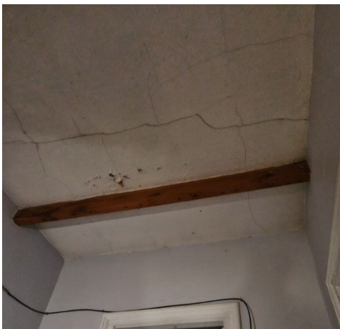
Figure 15: Parallel cracks to collar ties.
