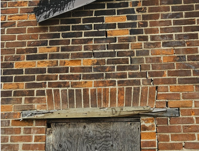
Figure 9: Diagonal cracking at openings.
