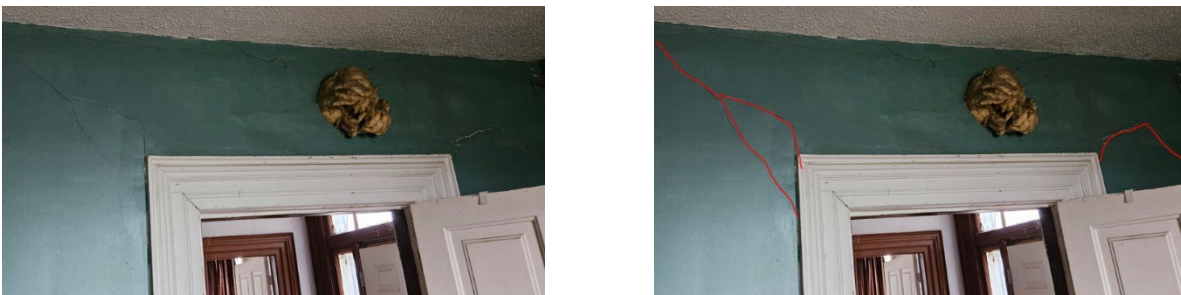
Figure 8: Floor beneath is deflecting considerably where partition walls are sinking and cracking as shown in red.
