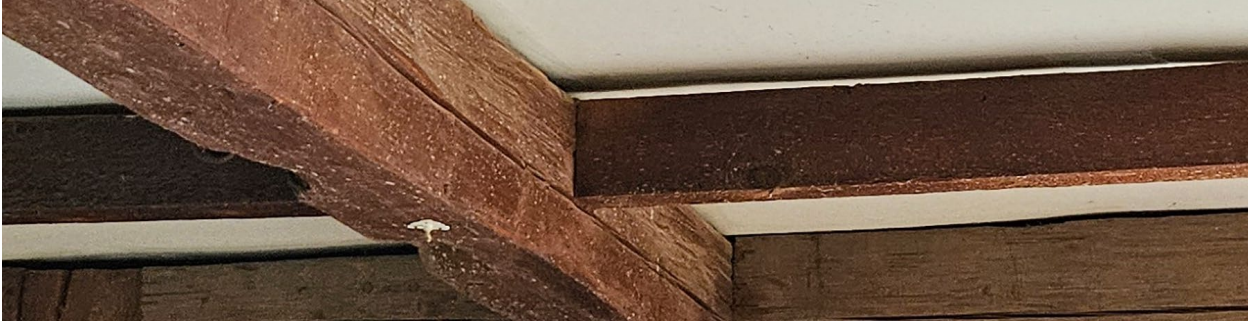
Figure 23: Deflection between ceiling and joists.
