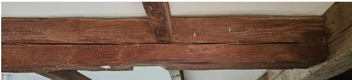
Figure 5: Structural main supporting beam undergone flexural bending failure with splitting from end-to-end.
