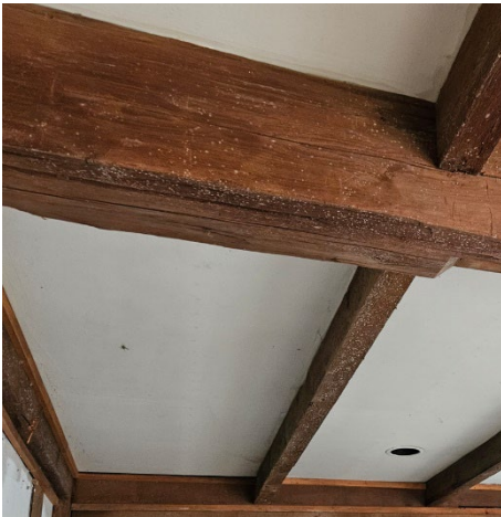
Figure 24: White mold seen throughout on timber and wood framing.
