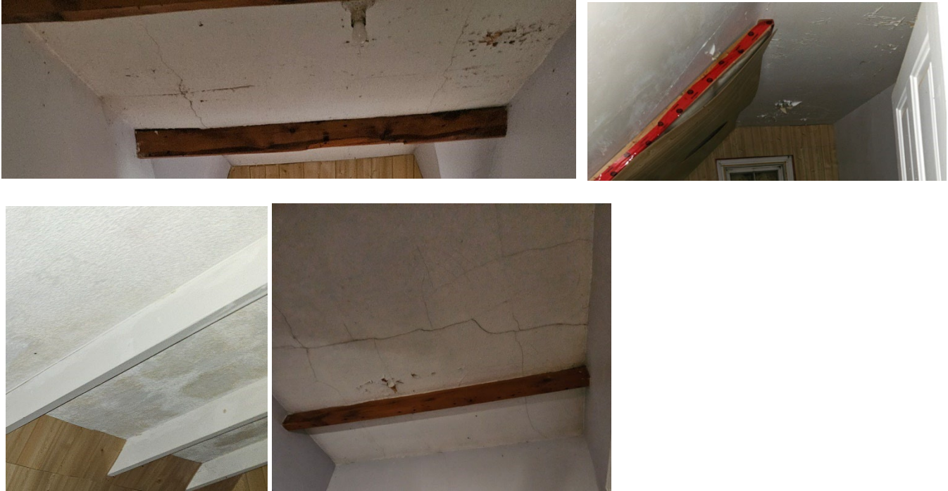
Figure 1: Cracking shown throughout the second floor ceiling and discolouring due to water penetration through roof.
