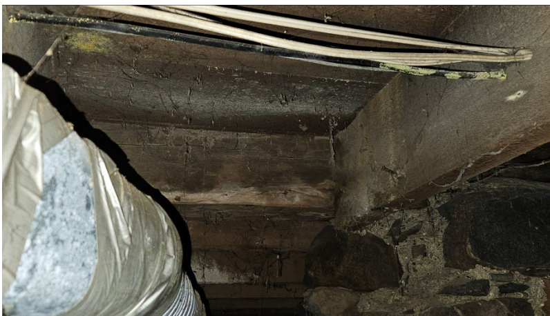
Figure 22: White mold and water discoloration due to water moisture and penetration.
