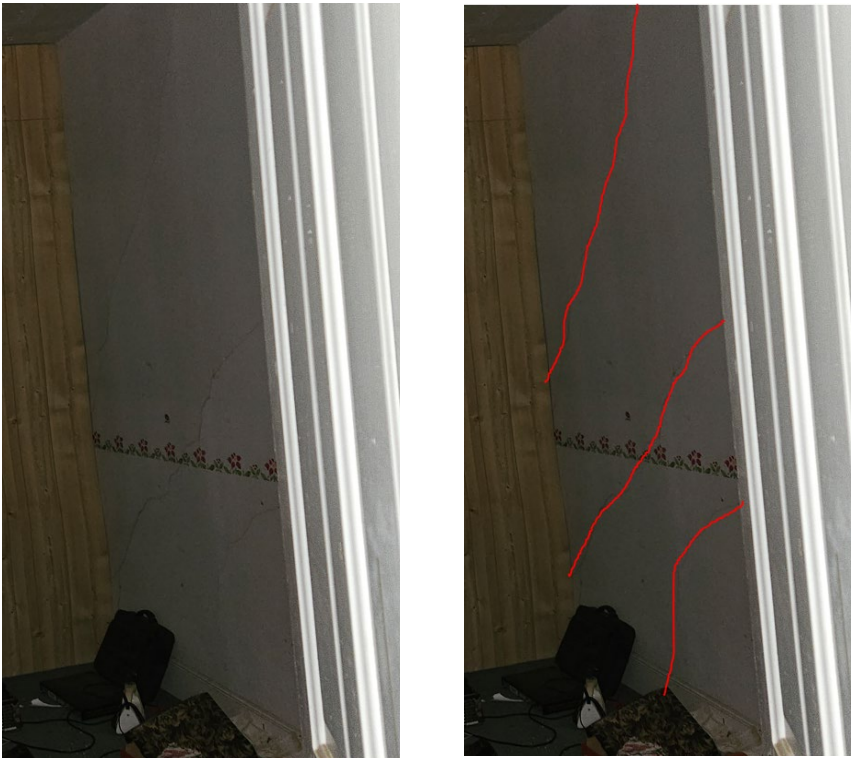
Figure 27: Diagonal cracking seen and may be from one side of building settling more than other side.
