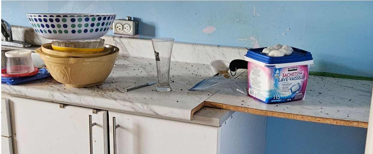
Figure 28: Droppings seen throughout the structure indicating infestation of rodent or wildlife.
