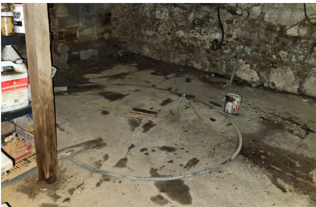
Figure 19: Discoloring of slab due to water absorption and infiltration.
