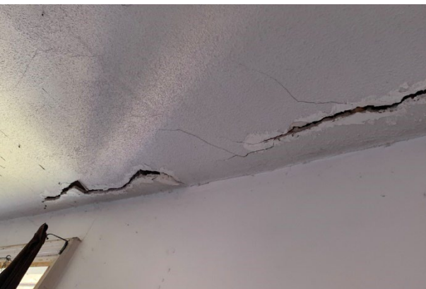
Figure 16: Ceiling tears at wall interface due to lateral displacement and walls pushing outwards out of plumb due to potential roof instability.
