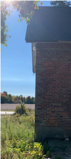
Figure 10: The east wall appears to not be plumb.
