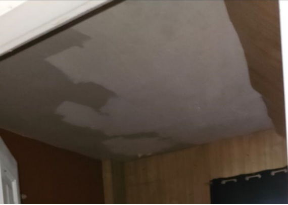
Figure 14: Ceiling work reworked (patched).
