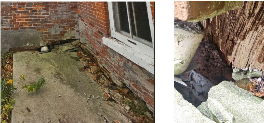
Figure 2: Exterior brick is crumbling throughout the building where openings as shown exposes the building to water infiltration and infestation.
