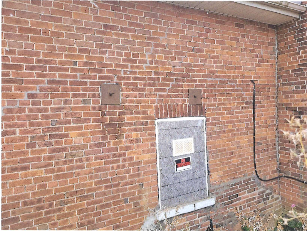
Photo 3 - View of North side showing steel plates and ends of steel cross ties at second floor, also cracking
