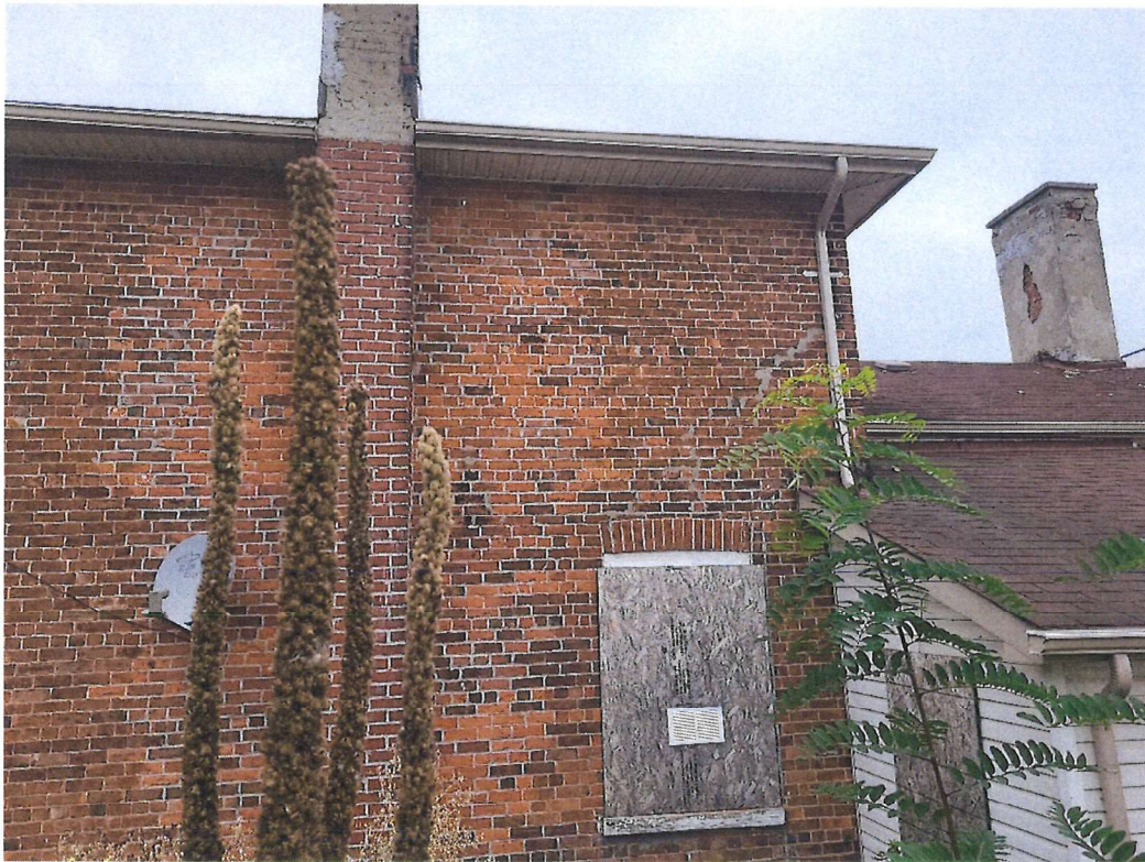
Photo 4 - View of South side showing cracking and evidence of repairs
