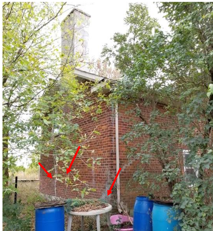
Figure 49: North and east façades of the East Wing. Note, extensive damage and repair to the east wall (red)
