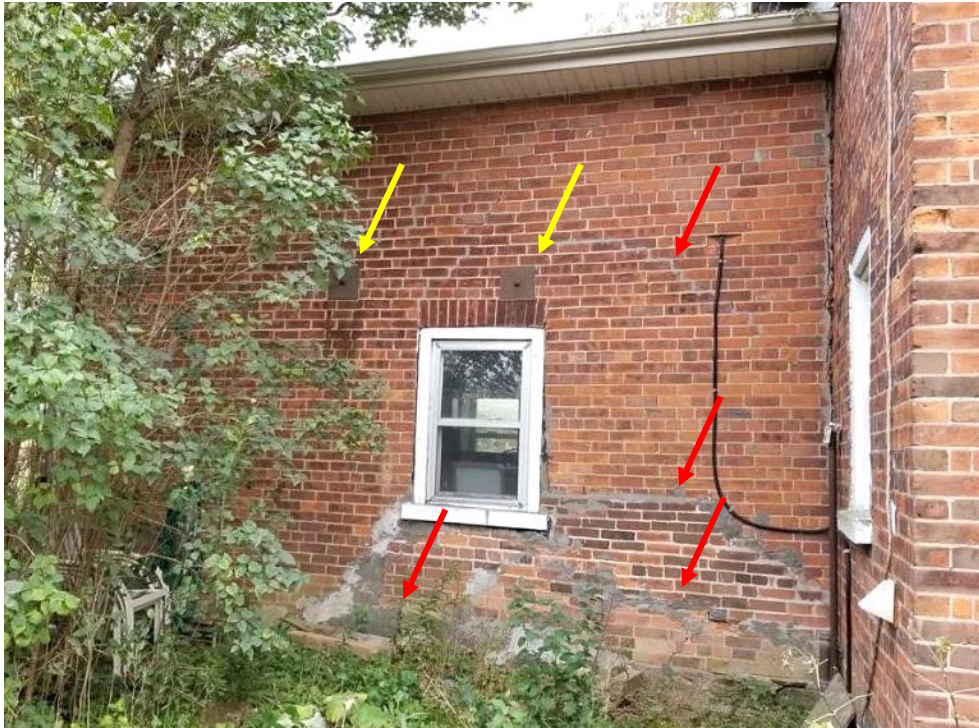
Figure 50: Extensive damage and repair to the north wall (red). Note the metal rods to secure the wall (yellow).
