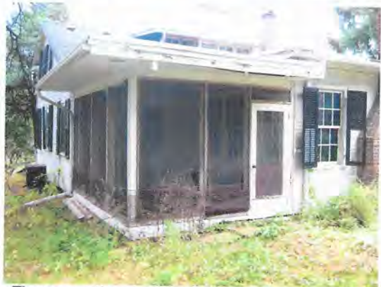
The connections between the 1825 house and later additions are not very sympathetic. Note deteriorated finishes.
