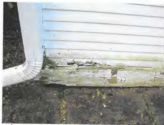
In some places at the base of building, there are signs of deterioration in the wood.
