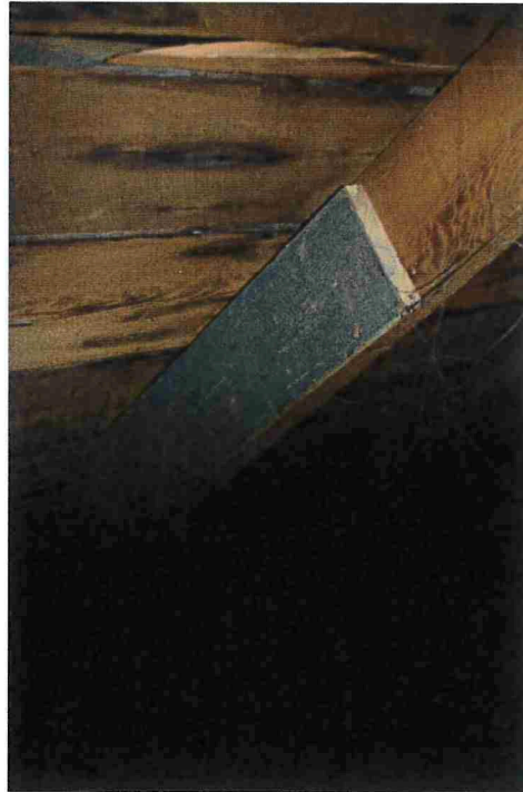
Figure 25: View of the roof construction as seen from the attic access (December 2016).
