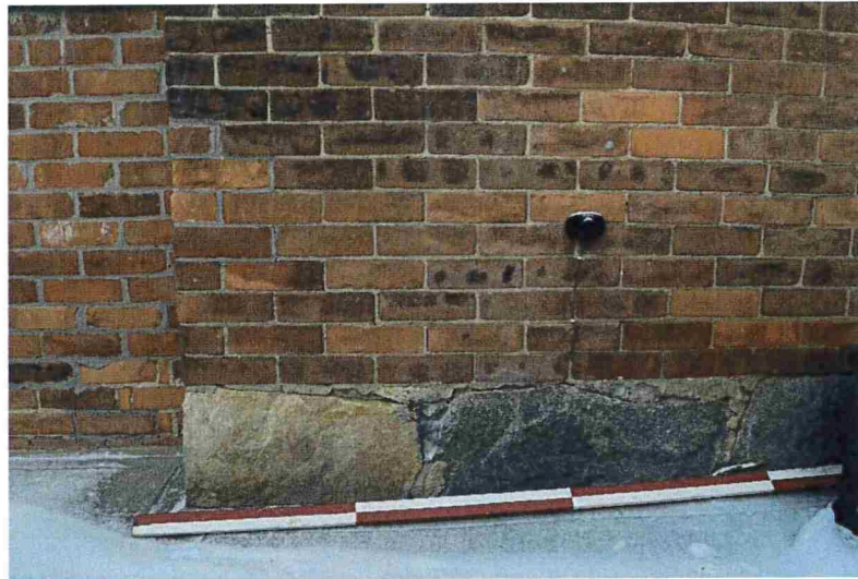
Figure 8: Random rubble fieldstone foundation and brick masonry at the southwest corner of the house (December 2016).
