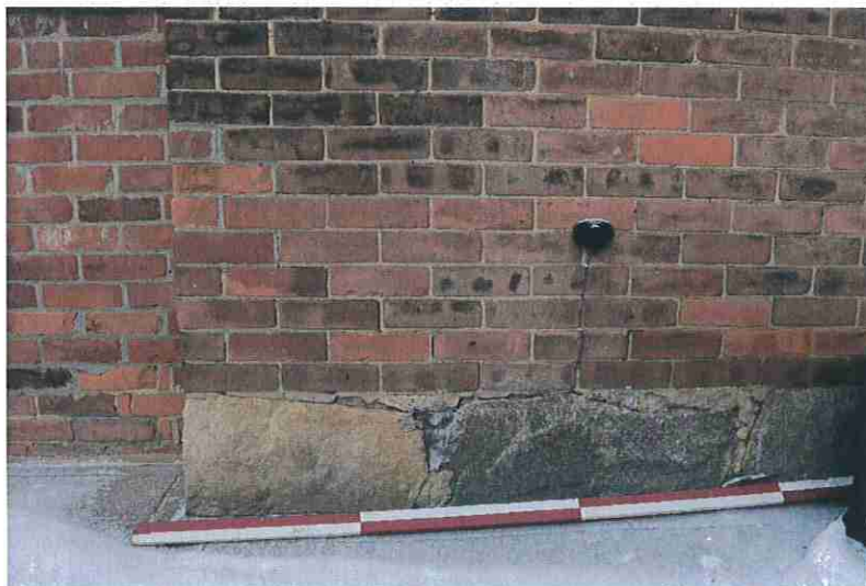
Figure 20: Random rubble fieldstone foundation and brick masonry at the southwest corner of the main block.
