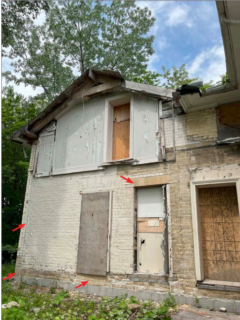
4. Bassingthwaite house, east elevation, on concrete block foundations and general site grading complete. New buff brick installed at the base and lintel, and brick repairs by DG Group.
