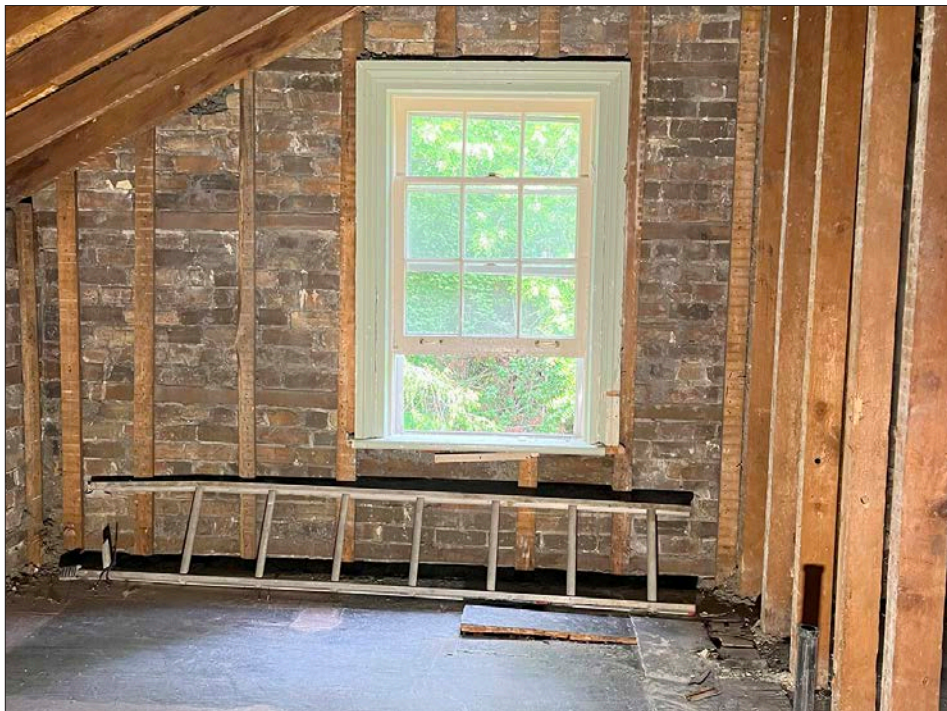
15. Basingthwaite house, second level, the existing roof and wall finishes are demolished, the perimeter brick wall, interior wall studs and roof joists are retained.
