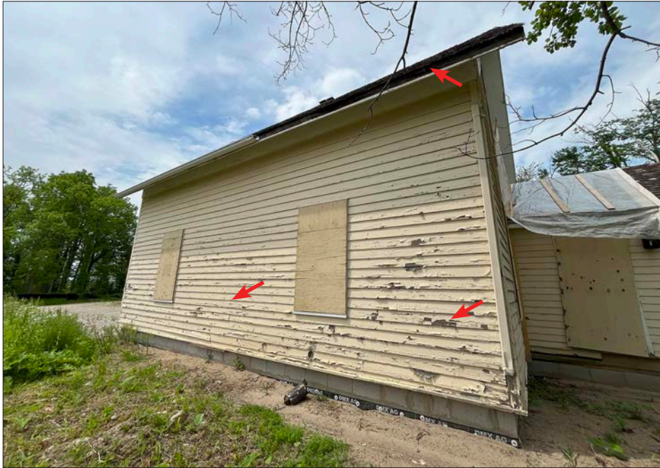
23. Munshaw house, east elevation, on concrete block foundations and general site grading complete. ERA noted that a section of the eaves-through has fallen off and more paint flaking on the facade.
