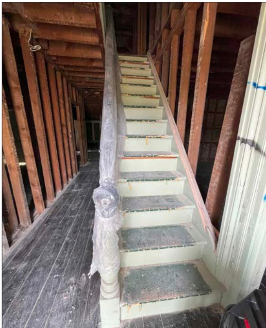
11. Basingthwaite house, ground level, the main stair newel post and handrails protected. The existing ceiling and wall finishes are demolished, the interior wall studs and floor joists are retained.
