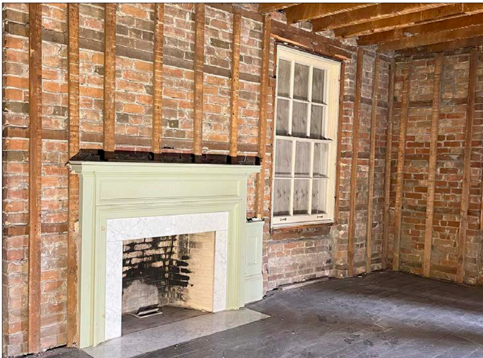
13. Bassingthwaite house, ground level, the existing floor and wall finishes are demolished, the perimeter brick wall, interior wall studs and floor joists are retained.
