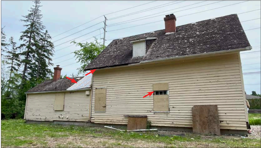
19. Munshaw house, west elevation, on concrete block foundations and general site grading complete. ERA noted the cedar shingles have deteriorated since the last site visit in 2021 and a section of the eaves-through has fallen off. ERA noted tarp protection installed at the roof and walls of the house. ERA recommends installing plywood over exposed opening.
