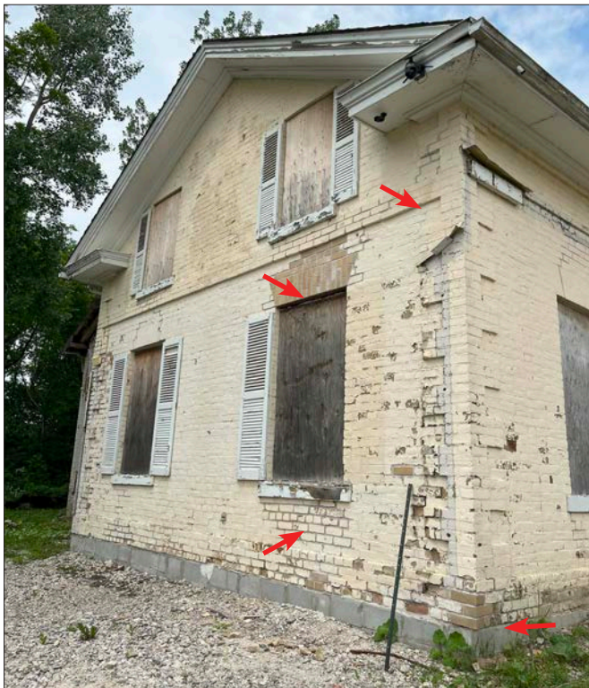
2. Bassingthwaite house, east elevation, on concrete block foundations and general site grading complete. New buff brick installed at the base and step cracking repairs by DG Group.
