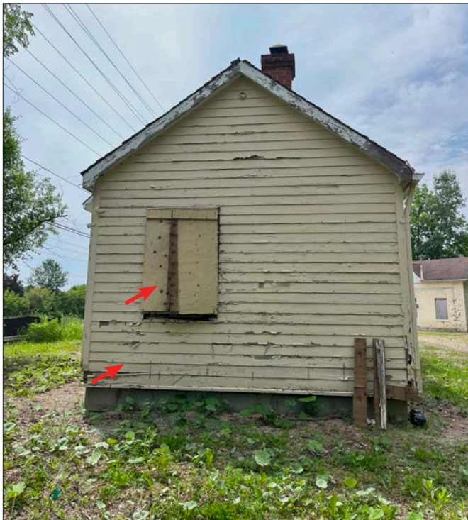
20. Munshaw house, north elevation, on concrete block foundations and general site grading complete. ERA noted more paint flaking on the facade. ERA noted the plywood installed over the opening is broken, ERA recommends installing new plywood.
