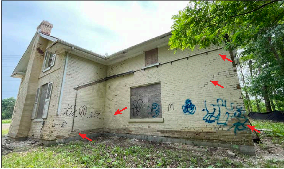
6. Basingthwaite house, west and south elevation, on concrete block foundations and general site grading complete. New buff brick installed at the base and step cracking repairs by DG Group. Graffiti on the facades is noted.
