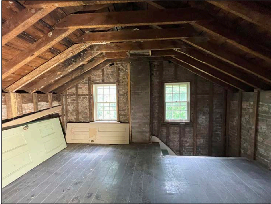
16. Bassingthwaite house, second level, showing the existing roof and wall finishes are demolished, the perimeter brick wall, interior wall studs and roof joists are retained. Original doors have been salvaged.
