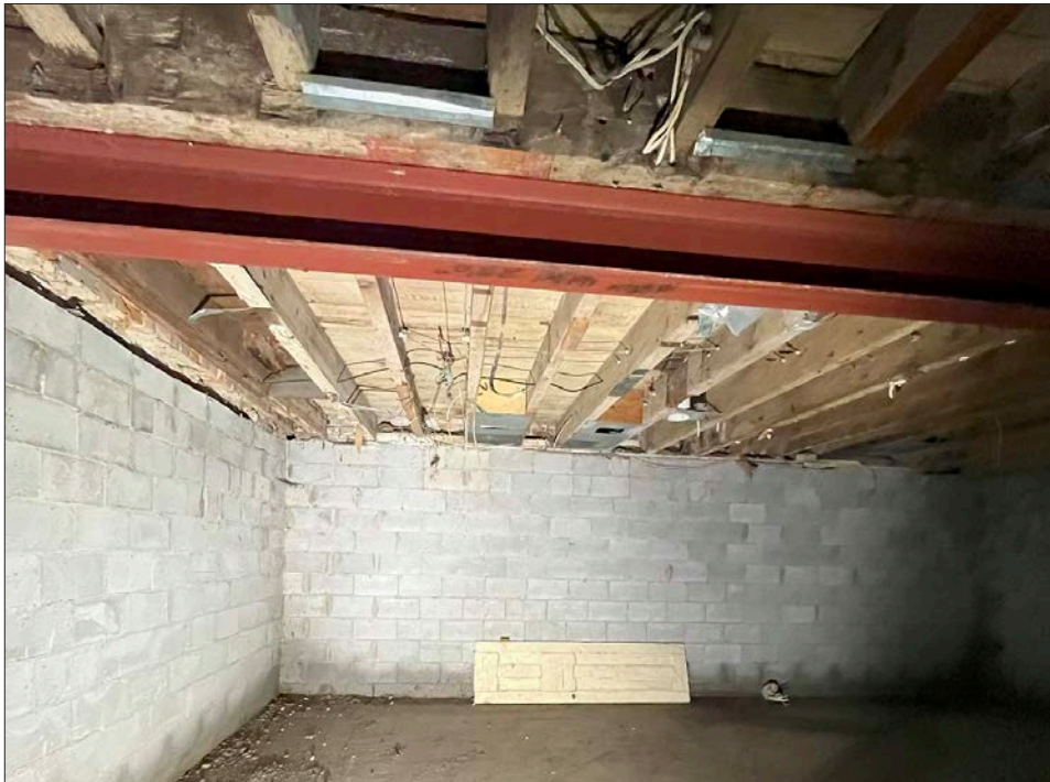
9. Bassingthwaite house, basement level, showing the concrete block foundation walls, concrete floor and steel structure.
