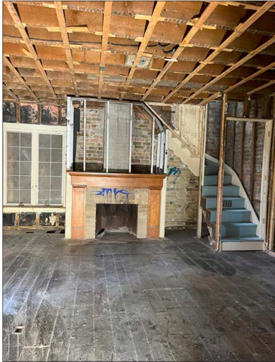
14. Basingthwaite house, ground level kitchen area, the ceiling and wall finishes are demolished, the perimeter brick wall, interior wall studs and floor joists are retained.
