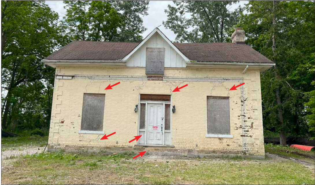
1. Bassingthwaite house, north elevation, on concrete block foundations and general site grading complete. New buff brick installed at the base, step cracking repairs and wood panel installation by DG Group.
