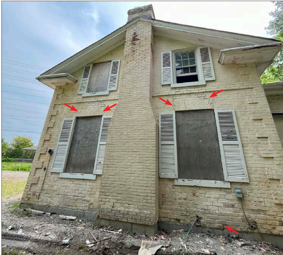
7. Basingthwaite house, west elevation, on concrete block foundations and general site grading complete. New buff brick installed at the base and step cracking repairs by DG Group.
