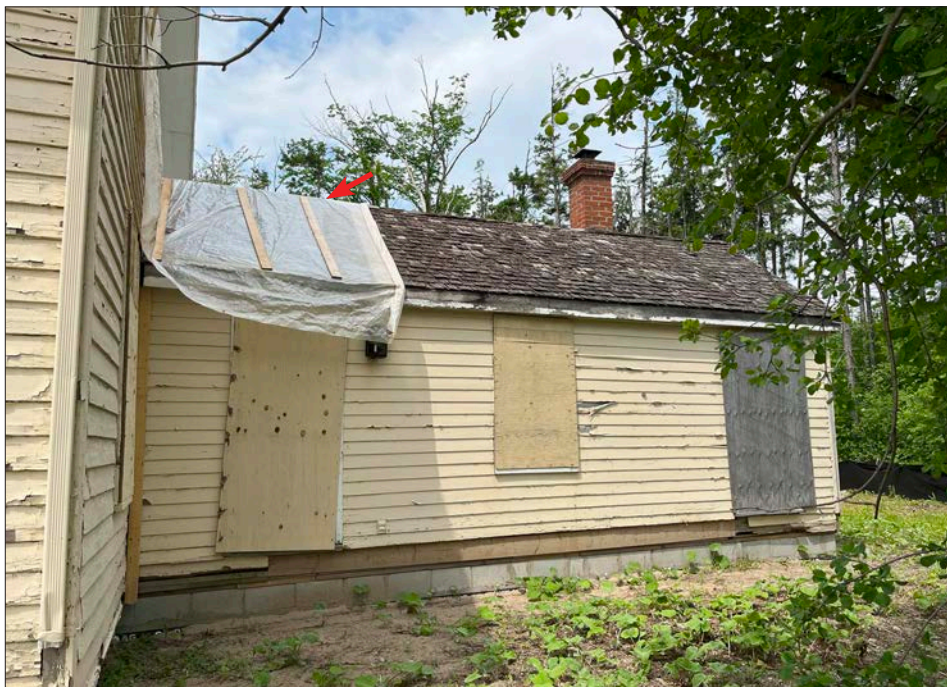
22. Munshaw house, east elevation, on concrete block foundations and general site grading complete. ERA noted the cedar shingles have deteriorated since the last site visit in 2021. ERA noted tarp protection installed at the roof and walls of the house.
