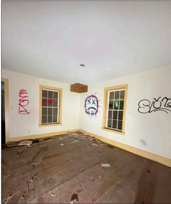
25. Munshaw house, ground level, no interior work completed. Graffiti on the walls is noted.
