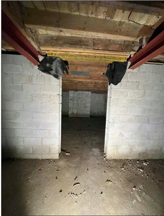
10. Basingthwaite house, basement level, showing the concrete block foundation walls, concrete floor and steel structure.
