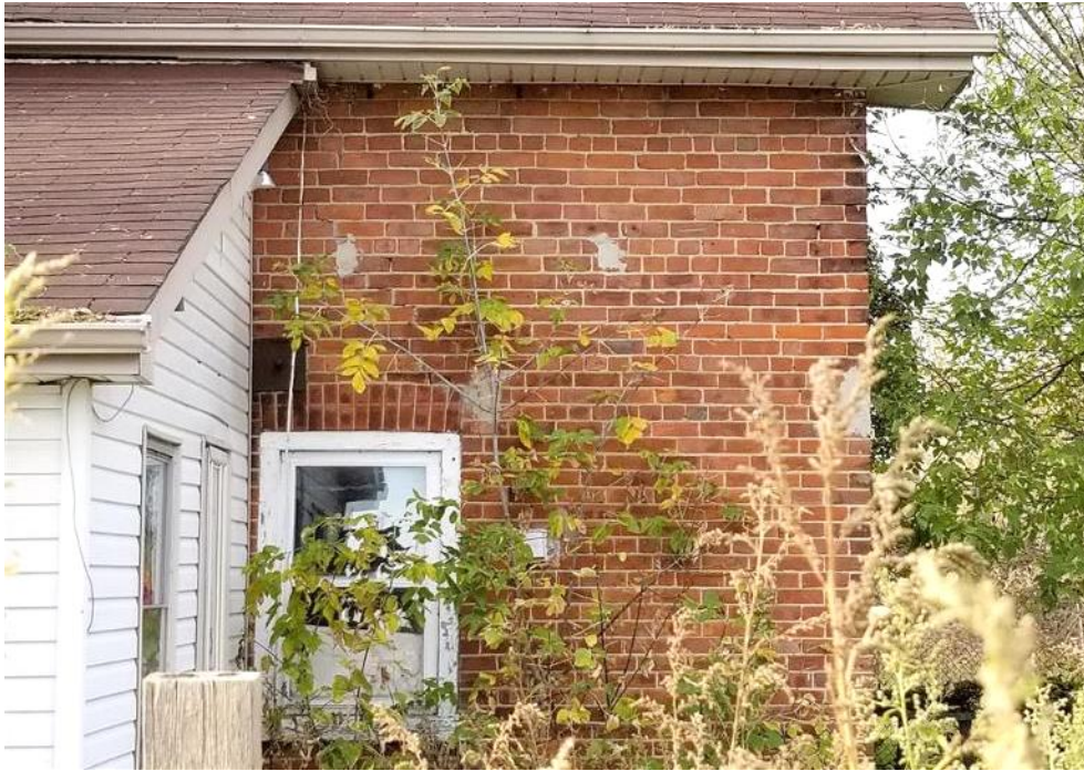
Figure 56: South façade of East Wing and east façade of the South Addition.
