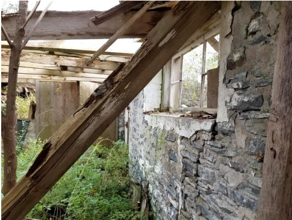
Figure 62: Interior of the collapsed barn.
