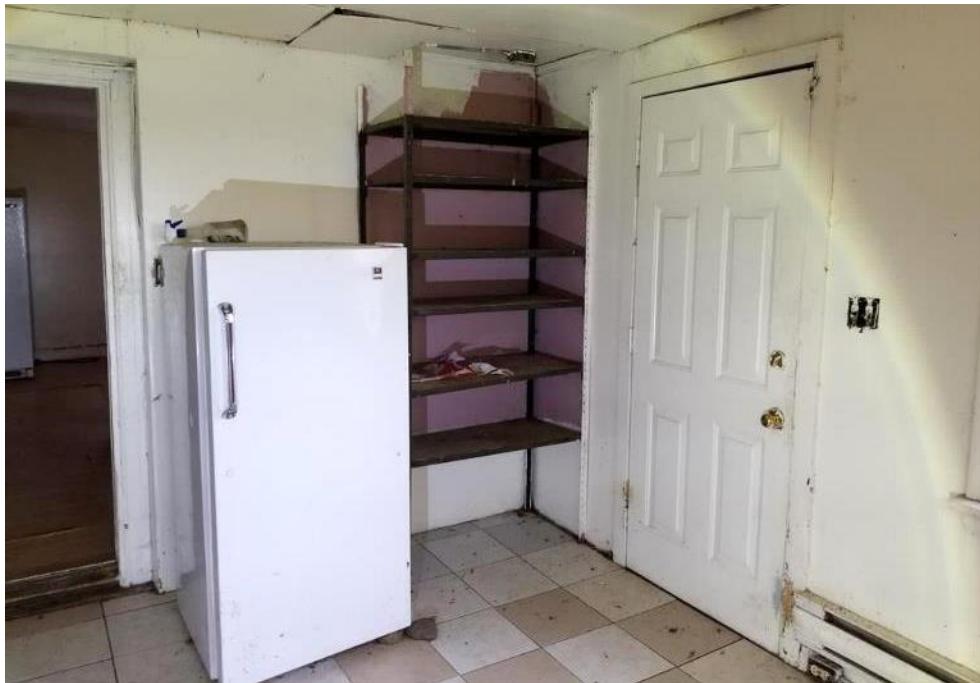
Figure 57: Facing northeast inside the South Addition with the exterior door on the east wall.
