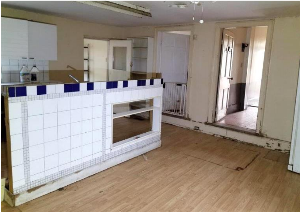
Figure 51: Interior of the East Wing facing west. Doorways to the Main Block to the west and South Addition to the south.
