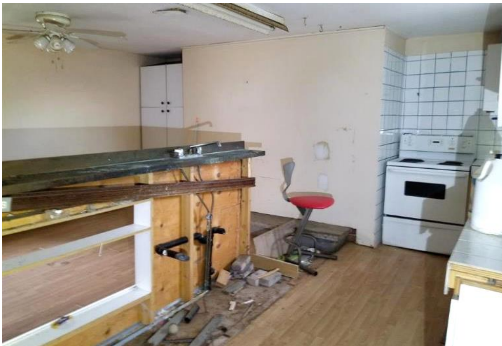
Figure 52: Interior of the East wing facing the east wall. Covered hearth in the centre of the wall.
