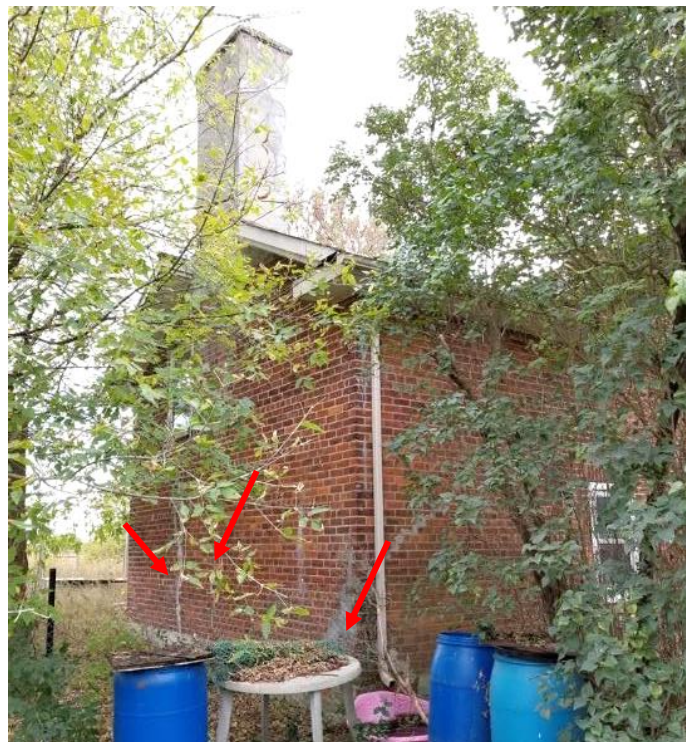
Figure 49: North and east façades of the East Wing. Note, extensive damage and repair to the east wall (red)
