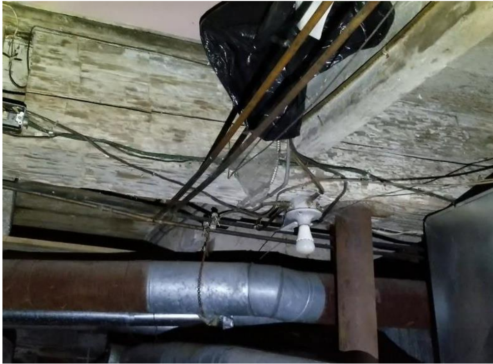
Figure 47: Close up of the summer beam running east-west across the basement ceiling.
