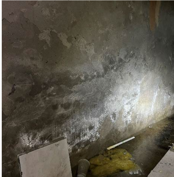
Bowing Wall (Parged with Concrete)
