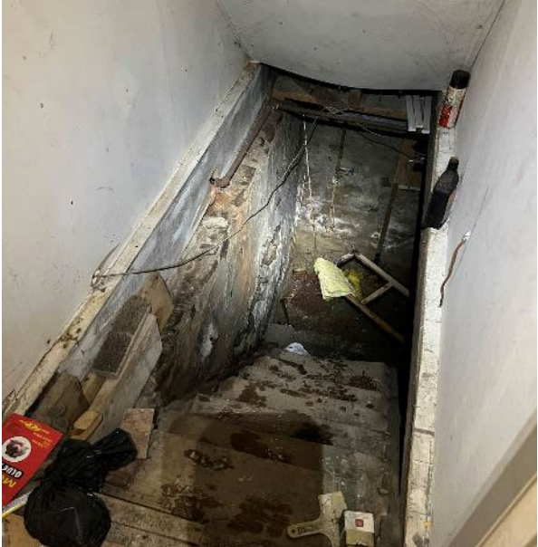
Basement Staircase (Damaged)
