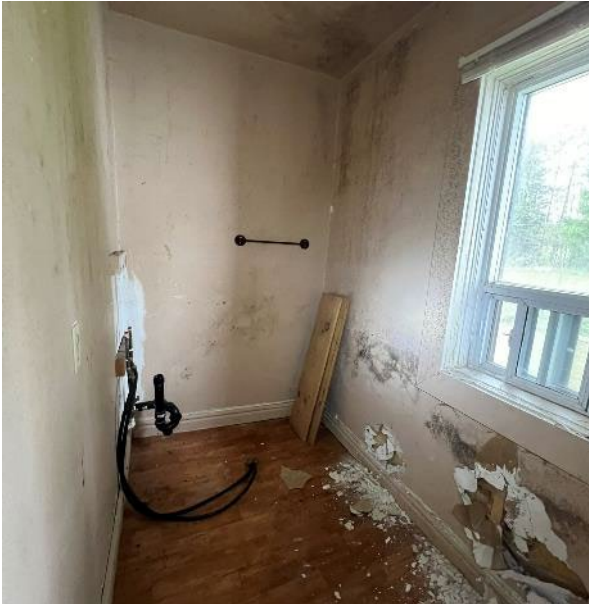
Mold, Drywall, and Animal Feces Damage
