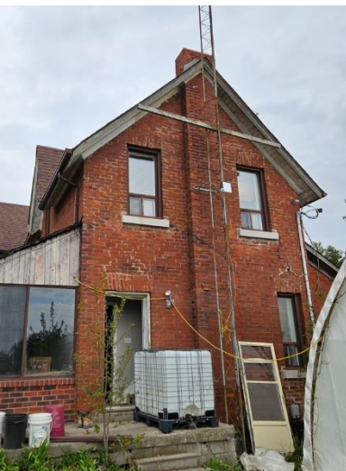
Figure. 17: East Chimney projected chimney with lack of interlocking and grouting to primary structure.
