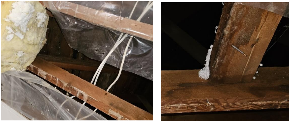
Figure 8: Roof sheathing appear wet and discoloured due to water penetration (left) ceiling joist and bridging member is discoloured due to water exposure (right)
