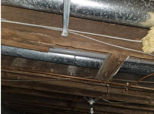
Figure 20: Floor joists cut, drilled and modified for mechanical works
