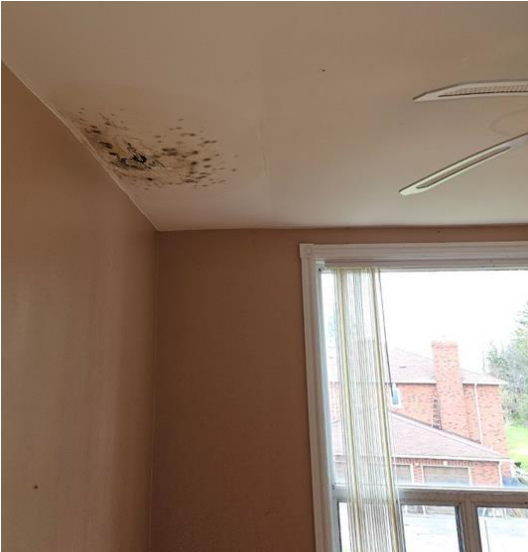
Figure. 16: Water damage/mold on the second-floor ceiling with fairly recent ceiling gypsum due to water leakage from roof.
