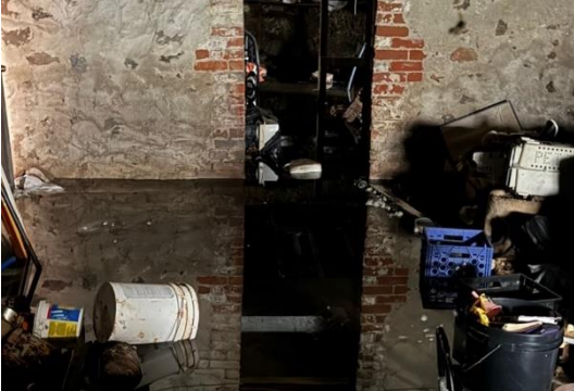
Figure. 11: Basement water leakage 1 to 2 feet high upon inspection.
