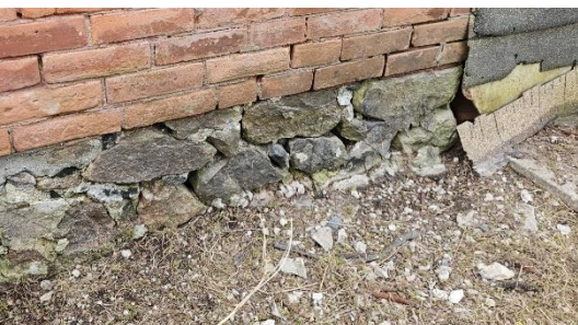
Figure 3: Load bearing foundation wall stones falling apart creating unsafe structural conditions and subject's basement to water leakage.
