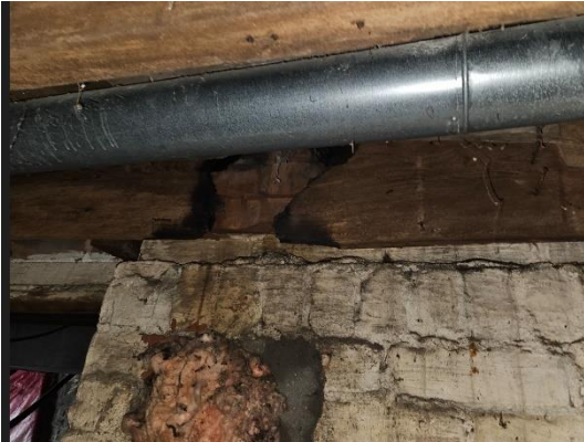
Figure 1: Evidence of Fire Damage impacting a ledger board carrying joists along basement foundation wall
