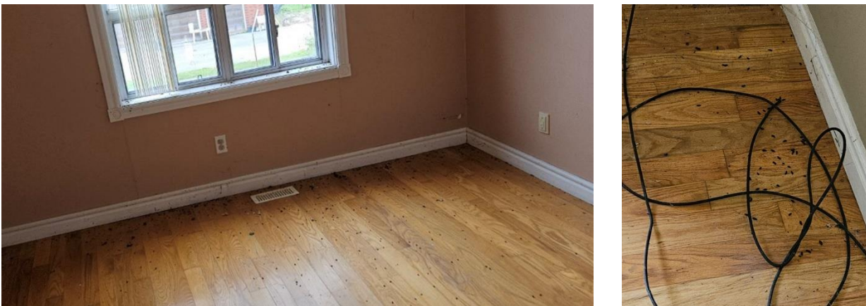
Figure. 15: Droppings and bug infestation on ground floor.
