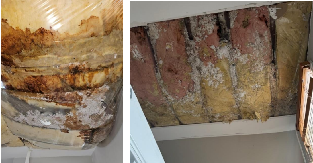
Figure 9: Discolouring of insulation from pink to brownish yellow and molding
