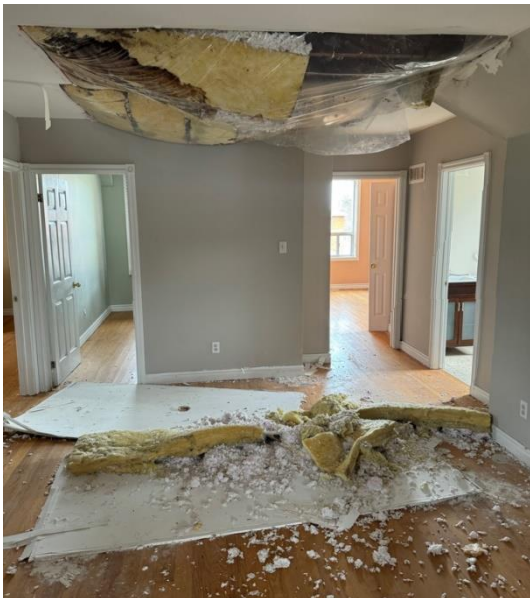
Figure 10: Ceiling collapsed due to possible excessive water wait from roof leakage.
