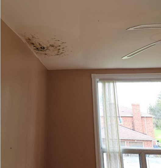
Figure. 16: Water damage/mold on the second-floor ceiling with fairly recent ceiling gypsum due to water leakage from roof.
