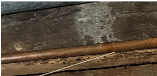
Figure 21: Bottom of floor joists appear to have termite markings.
