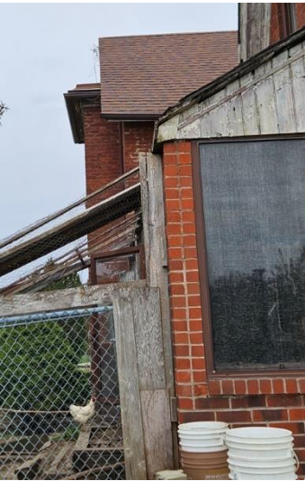
Figure 5: Left most walls are not vertically plumb and is leaning in towards itself
