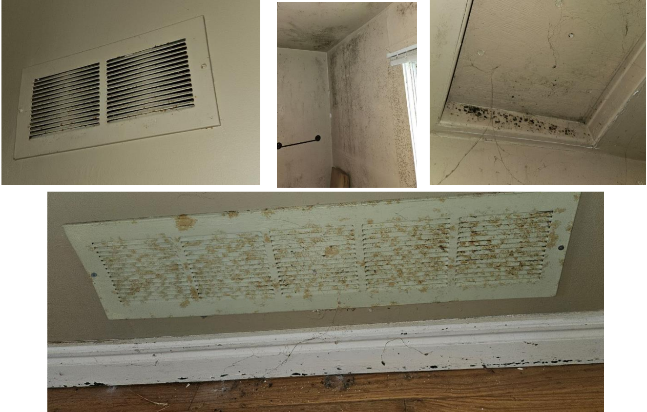
Figure. 14: Mold in vents, walls and ceiling throughout ground floor.
