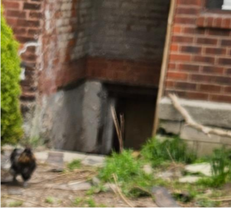
Figure 4: Walkout basement unreinforced wall subjected to lateral soil loading with soil beneath the slab addition on the south east corner of structure
