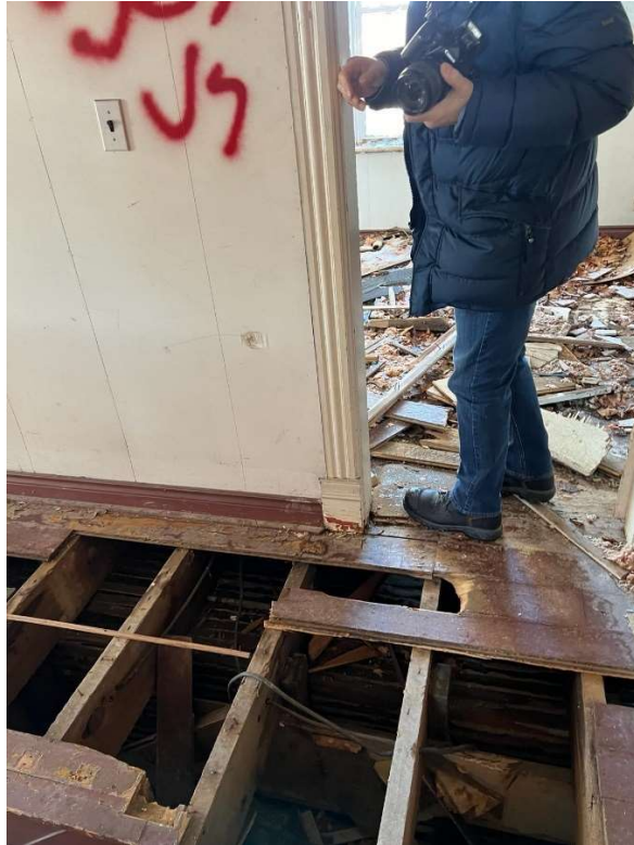
Pic. 19: Broken Floor, Debris, and Deterioration
