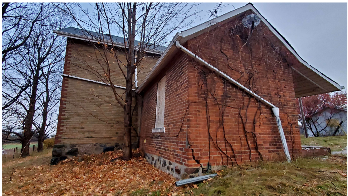
Pic. 7: Wide and large Vertically Inclined Crack in the Foundation and Brick Wall at Southeast Corner
