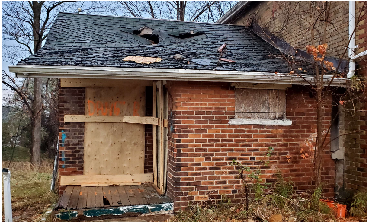
Pic. 10: Roof Caved In, Heritage House Backside- Part North face
