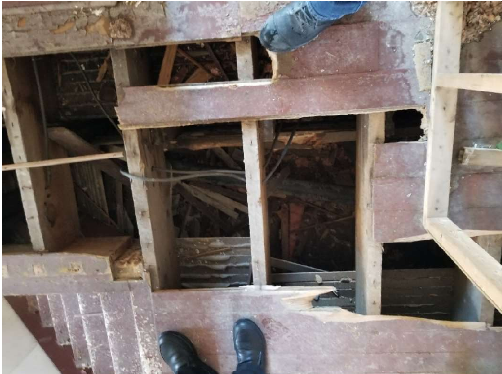
Pic. 20: Broken Floor, Debris, and Deterioration
