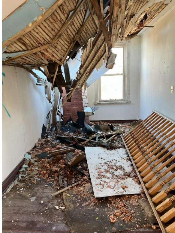
Pic. 14: Damaged Roof structure, Debris, Damp Wood Floor showing Decay and Deterioration
