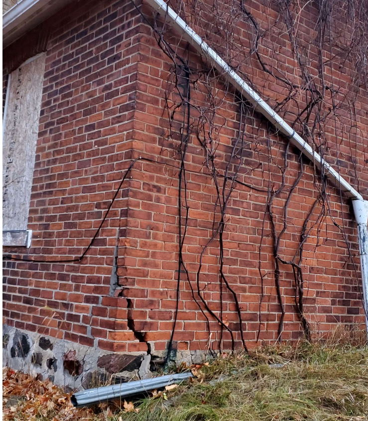
Pic. 8: Wide and Large Crack-Closeup
