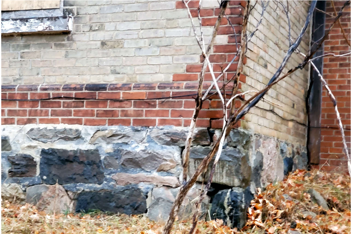
Pic. 6: Large and Wide Crack Closeup, Southeast Corner
