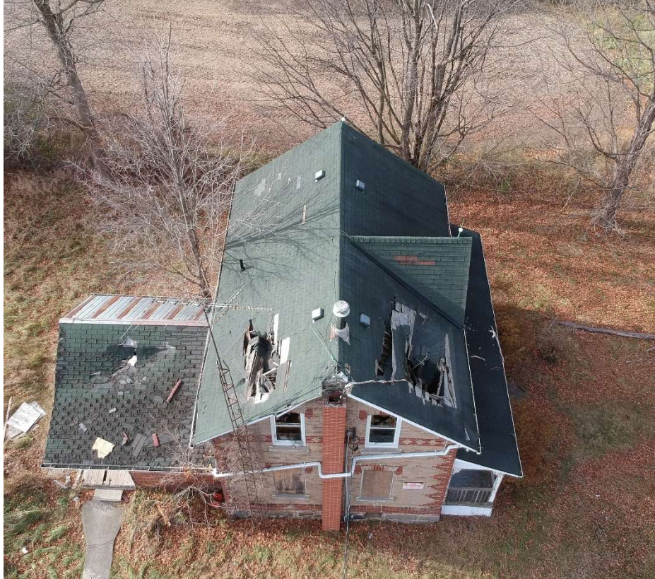
Pic. 12: Damaged Roof structure – Aerial View 1
