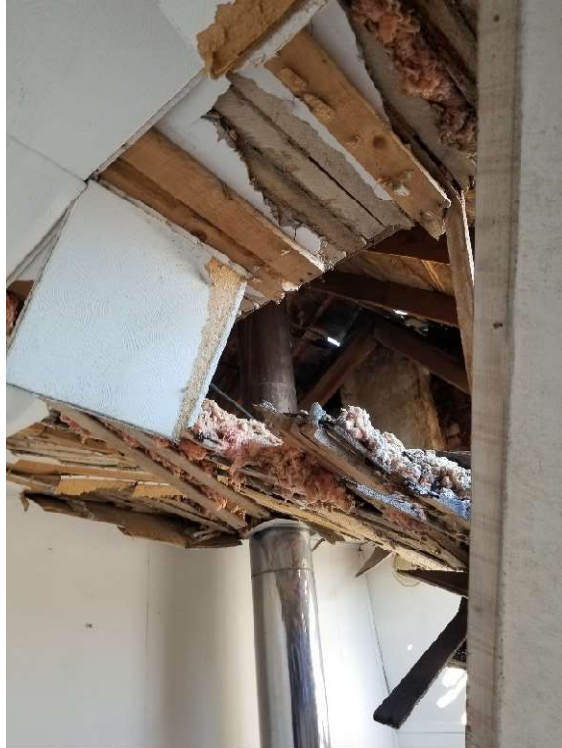
Pic. 16: Collapsed Ceiling with broken framing showing Deterioration
