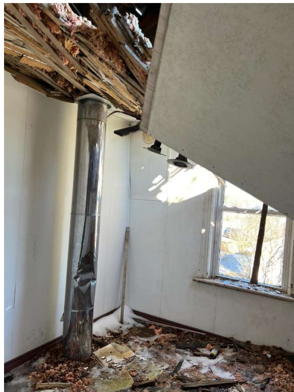
Pic. 15: Damaged Roof, Damp Wood Floor showing Decay and Deterioration
