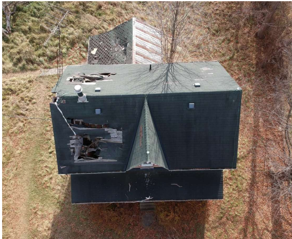
Pic. 13: Damaged Roof structure – Aerial View 2
