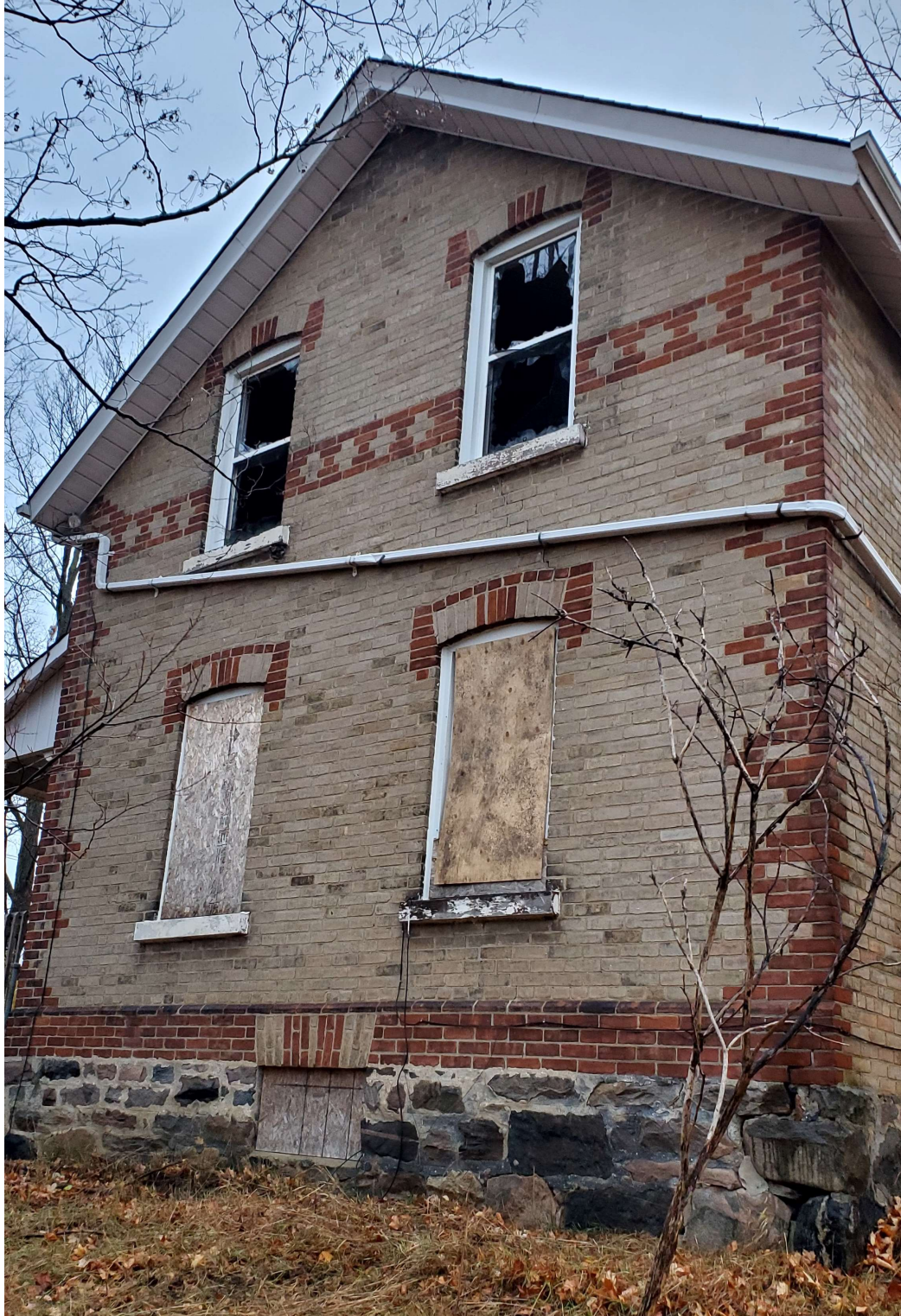
Pic. 5: Wide Large Crack in the Field Stone Foundation Wall at Southeast Corner
