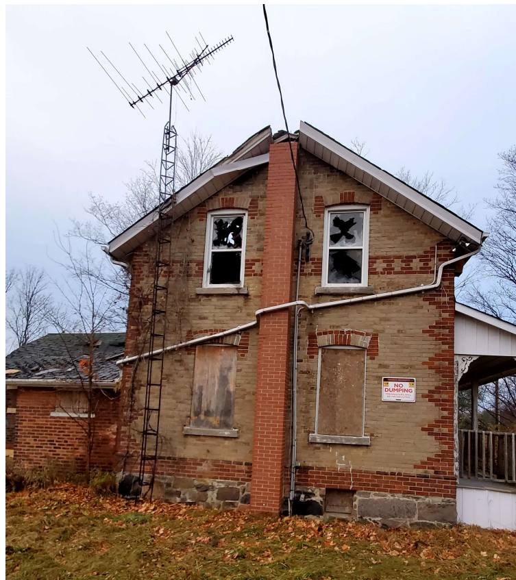
Pic. 11: Brick Chimney Broken from Top - North face
