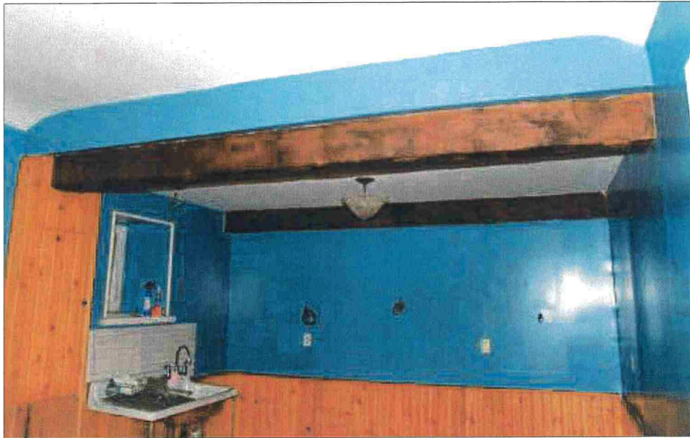
Figure 26: Interior of the stone portion of the rear wing showing the widely spaced and hewn ceiling joists.
