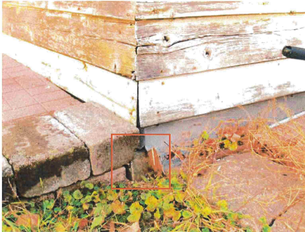
Figure 28: Poured concrete foundation evident at the southwest corner of the wing's wood section.
