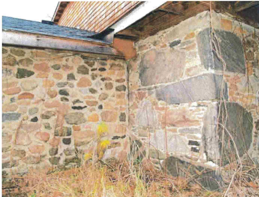
Figure 24: View facing northwest of the junction of the wing and original masonry near at the southeast corner of Joshua Oliver House. Note the contrast in stonework between the original construction on the right and the more recent wing construction on the left.
