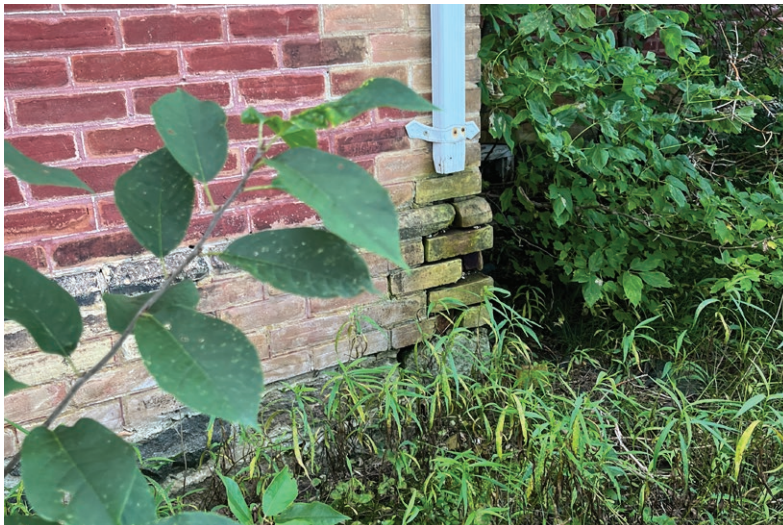
Dislodged bricks and missing downspout on the north elevation of the main farmhouse (ERA, 2023).
