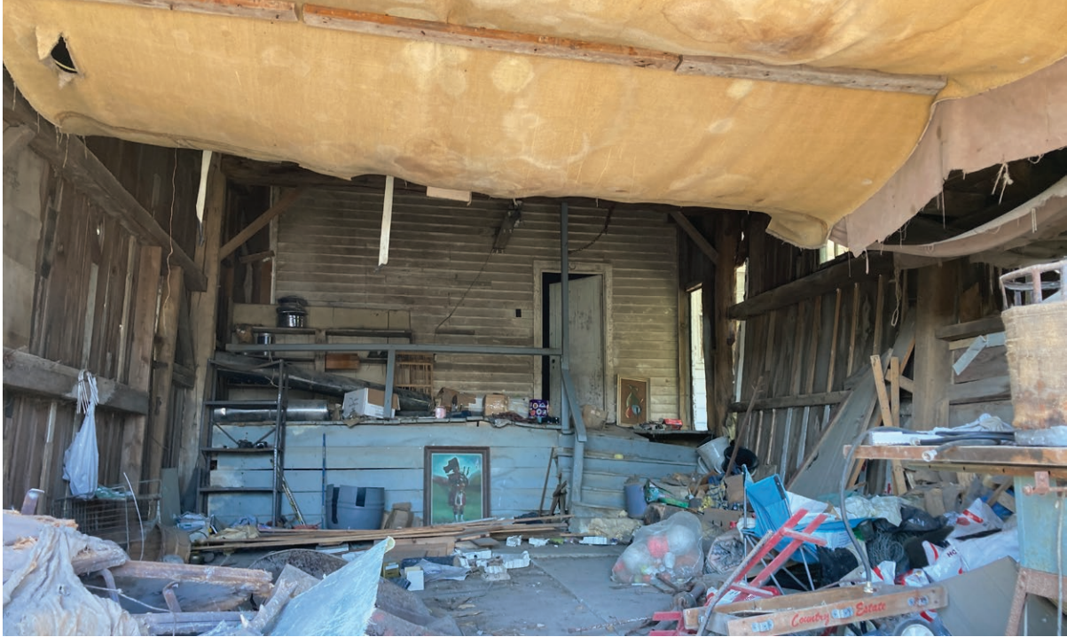
South elevation of the one-and-a-half-storey rear (original) farmhouse, obscured by the garage (ERA, 2023).
