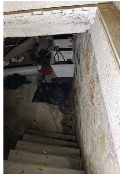
Defective concrete floor in the basement (ERA, 2023).
