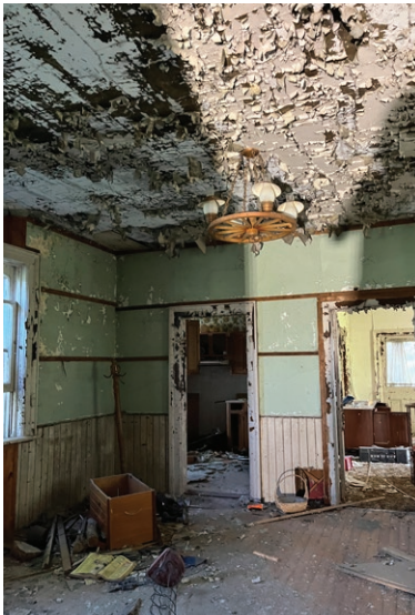
Mold, paint flaking, and plaster deterioration on the first floor (ERA, 2023).
