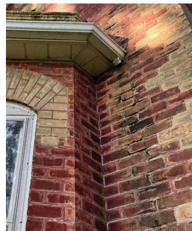
Brick staining on the east elevation of the main farmhouse (ERA, 2023).
