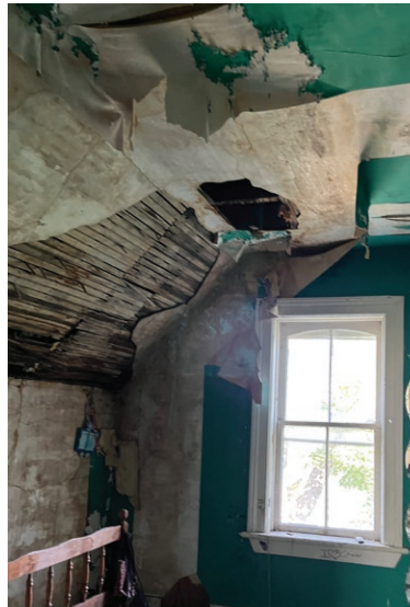
Ceiling deterioration on the second floor (ERA, 2023).
