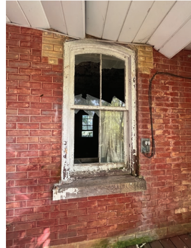
Broken window glass on the south elevation of the main farmhouse (ERA, 2023).
