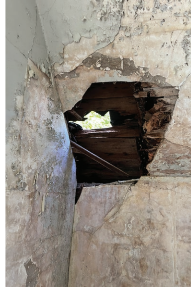
Missing roof boards at the top of the stairs on the second floor (ERA, 2023).
