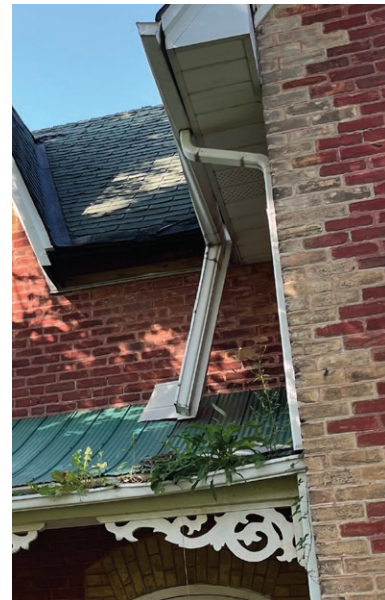
Detached gutter on the east elevation of the main farmhouse (ERA, 2023).
