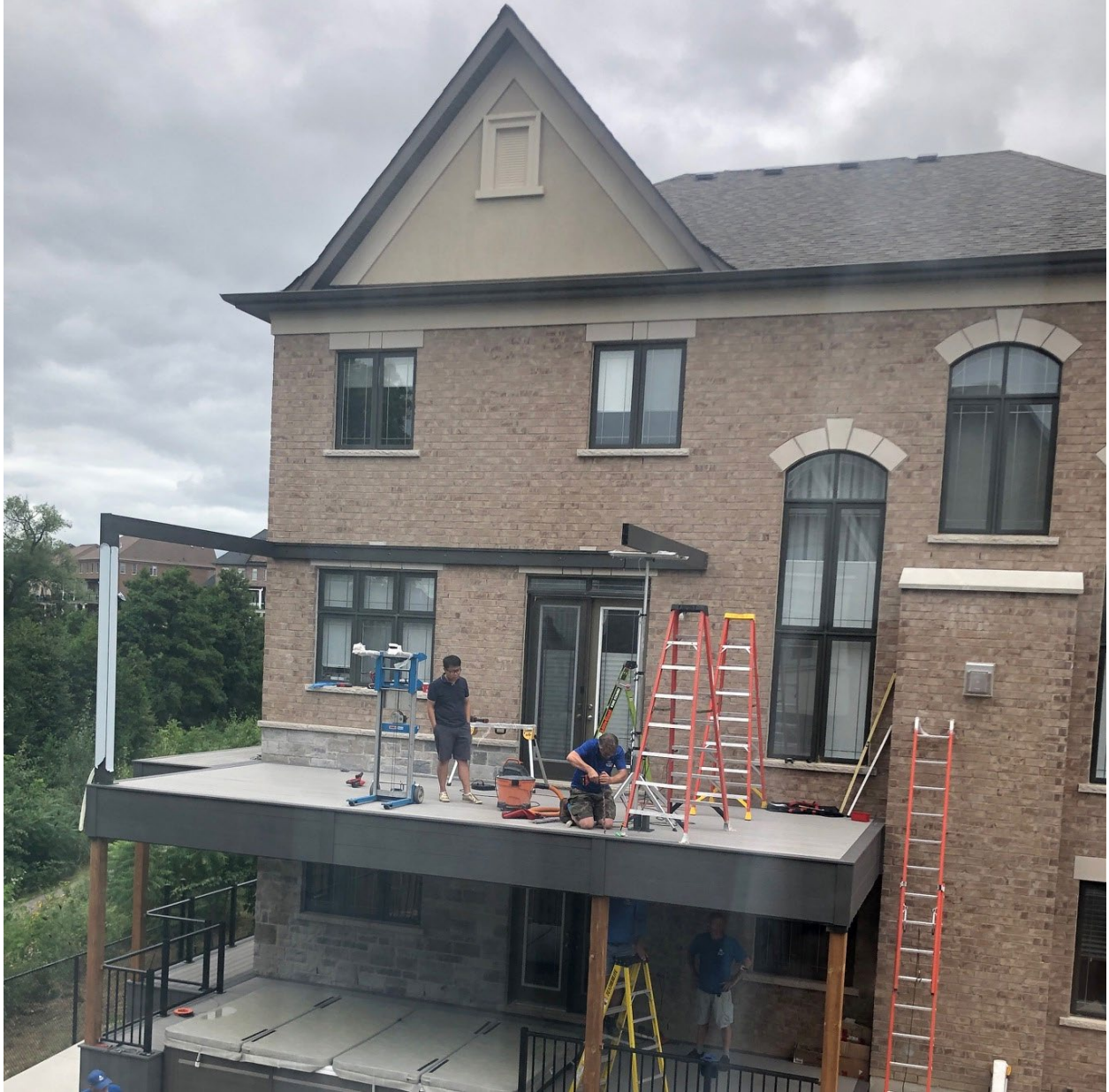
Illustration of size of the deck, proximity to rear property line, and the obstructed view being created on the left hand side as a result of the pergola and the decking on the side of the house.
