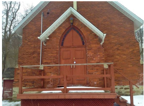
Figure 11. Front porch with doors reported to be saved from the fire. Entry stairs and deck is not original.
