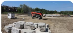
Example of a site in Vaughan undergoing alteration in preparation for development
