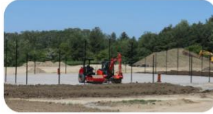
Example of a site in Vaughan undergoing alteration in preparation for development
