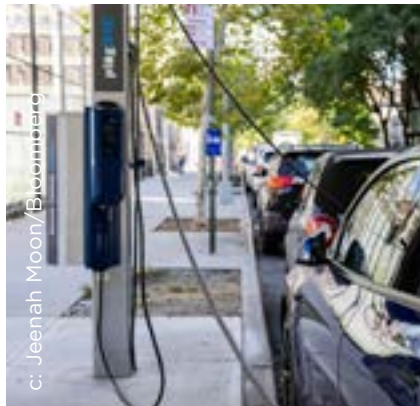
Figure 4.27. EV charging in parking lane.
