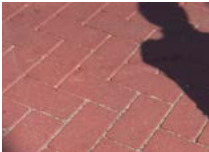
Figure 2.37. Material selection should consider context along with durability and life cycle cost.
