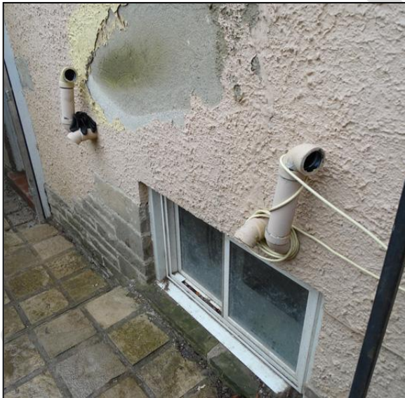
Figure 16: Left and Below: North façade showing concrete parging with a plaster topcoat, 2016
