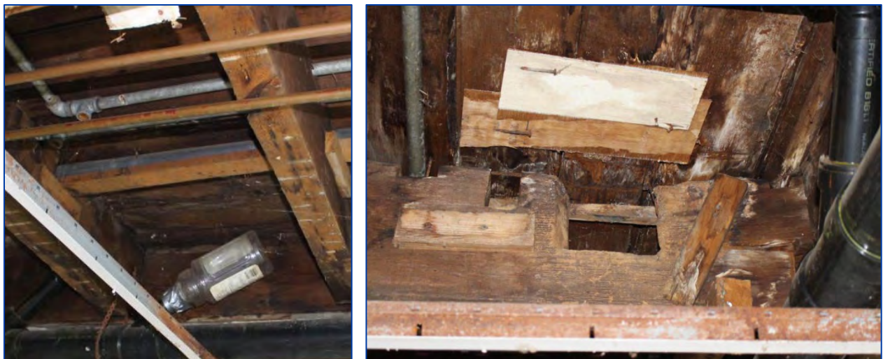
Figure 34: Ceiling in kitchen, located under bathroom
