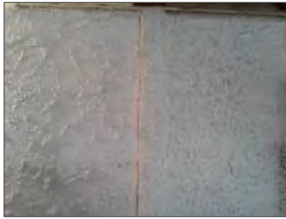
Photo 1: Texture coating on drywall walls throughout the first and second floors of the building.
