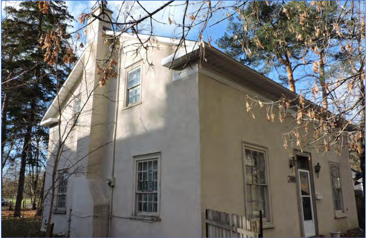
Figure 27: View northwest at the front façade and side elevation of the house on the Property
