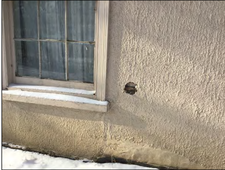
Photograph 8: Exposed exterior lathe on east elevation
