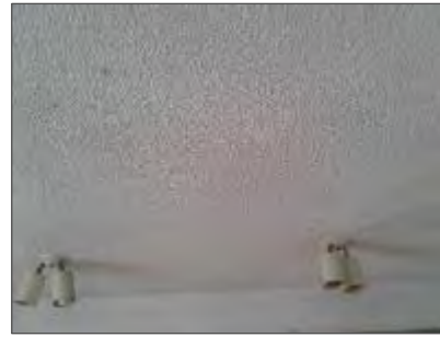
Photo 2: Texture coating on drywall and plaster ceilings throughout the first and second floors of the building.
