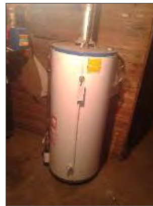
Photo 6: Domestic hot water tank insulated with non-asbestos fibreglass in the Basement (Loc. 7).
