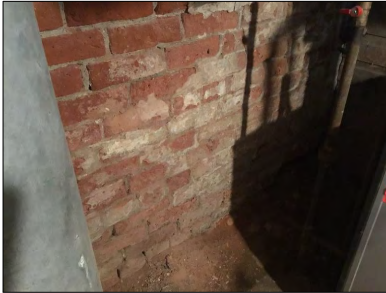
Photograph 7: Exposed brick foundation
