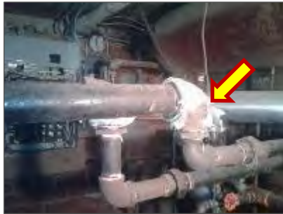
Photo 3: Asbestos containing paring cement on an elbow fitting in the Basement (Loc. 7).
