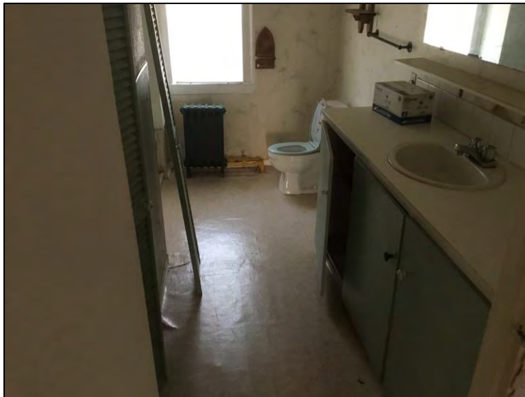
Photograph 2: Bathroom floor deflection
