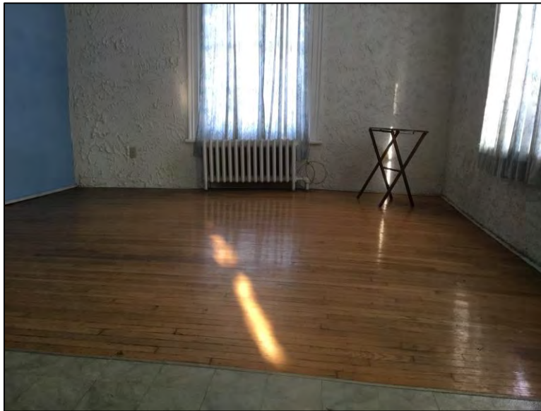
Photograph 3: Northeast living room floor deflection
