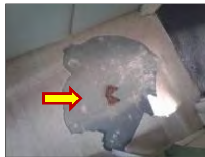
Photo 15: Asbestos containing 9" x 9" green vinyl floor tiles in the Bathroom and Laundry Room (Loc. 6).
