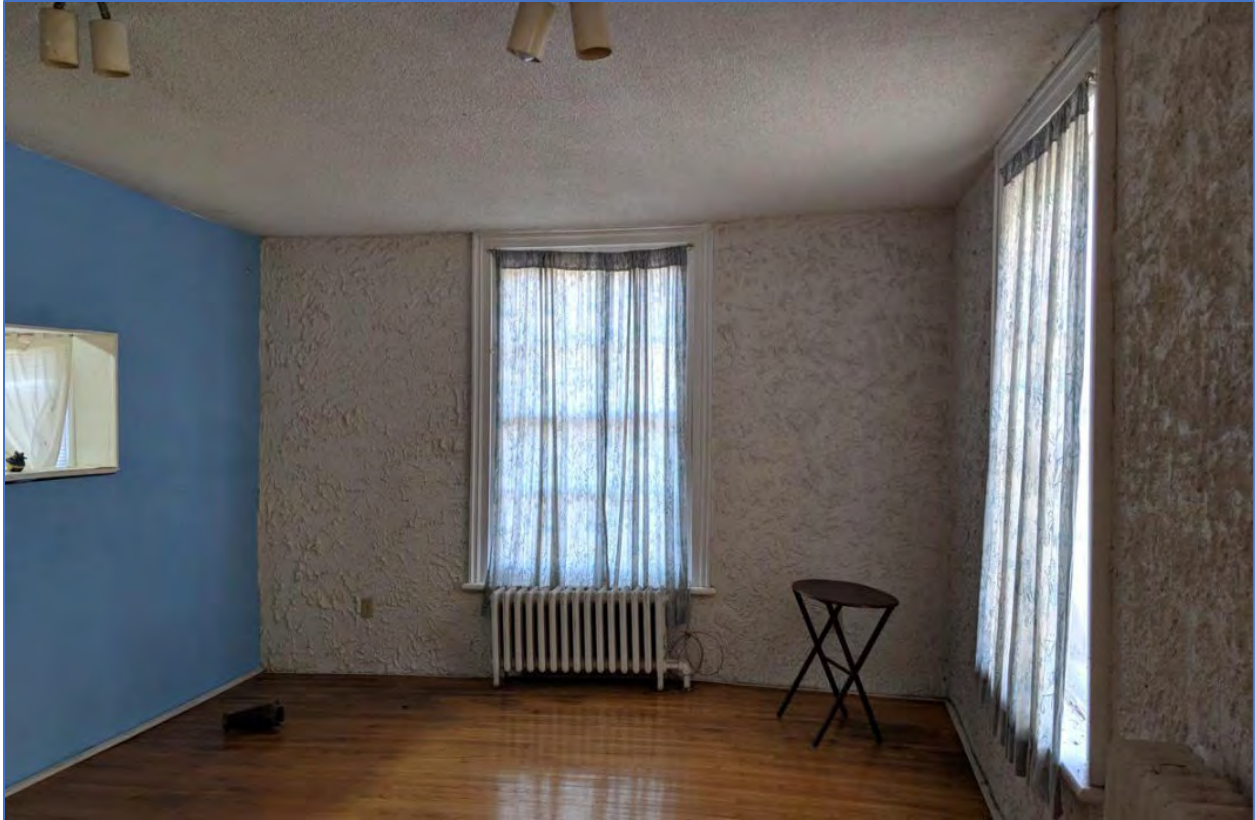
Figure 39: Dining area. Note the significant bow in the floor.
