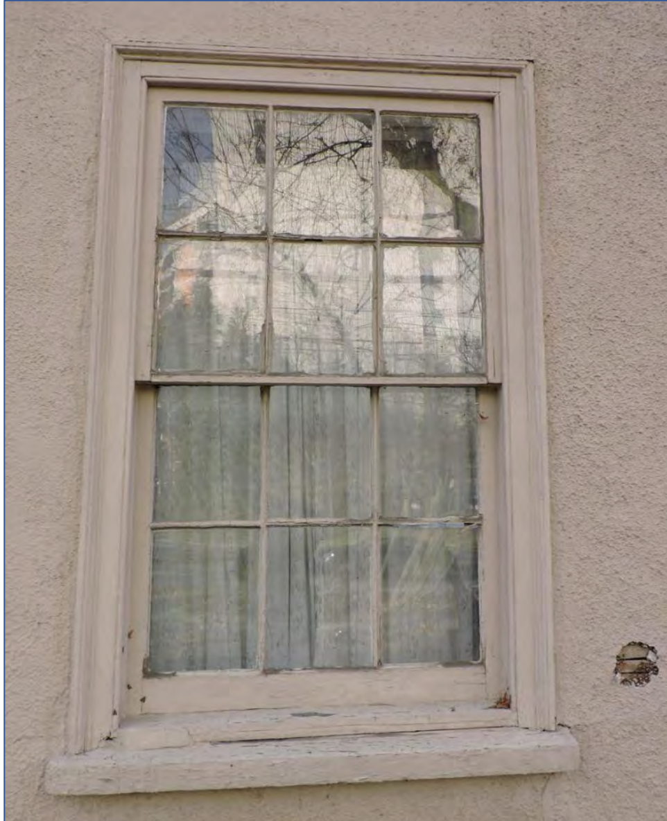
Figure 28: Detail view of a 6 over 6 double hung sash window, stucco finish on the wall and exposed circle showing lath and plaster cladding
