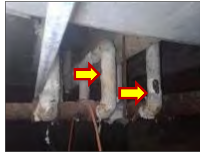
Photo 4: Asbestos containing aircell insulation on straight sections of piping in the Basement (Loc. 7).
