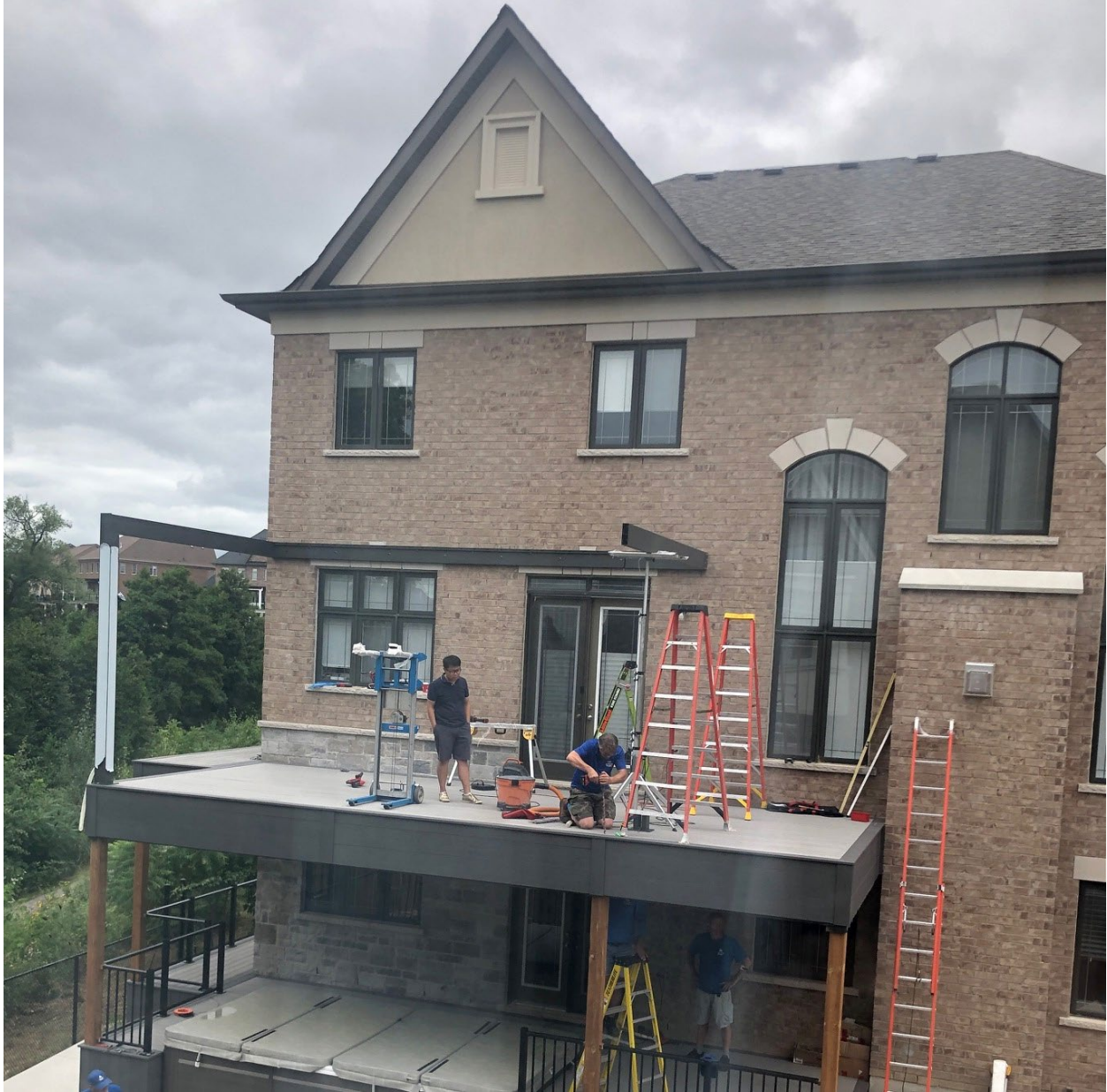
Illustration of size of the deck, proximity to rear property line, and the obstructed view being created on the left hand side as a result of the pergola and the decking on the side of the house.
