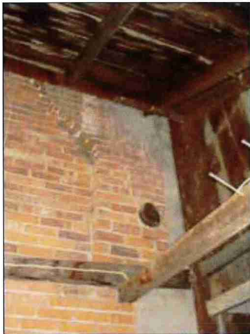
Photograph No. 39 Shed facing tail wing wall near garage door showing bricked in opening.
