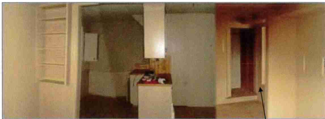
Photograph No. 36 Tail wing – ground floor kitchen – west wall (looking towards shed).
