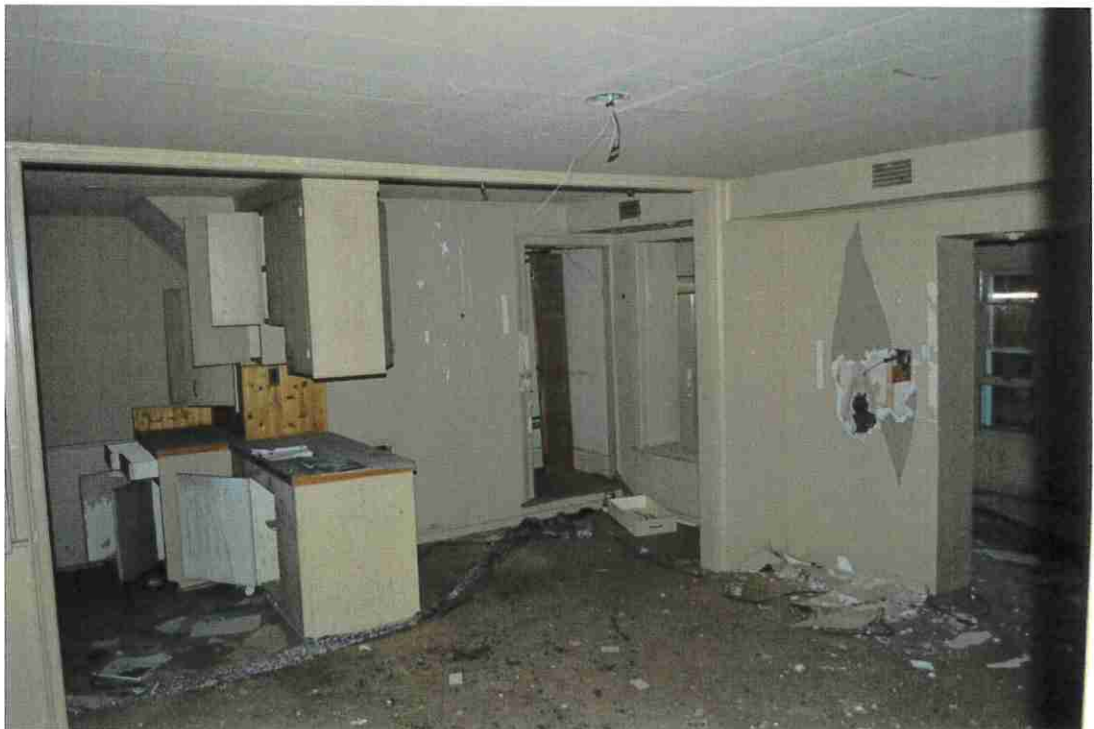
Figure 50: Ground floor of brick rear addition looking north west to enclosed north porch.
