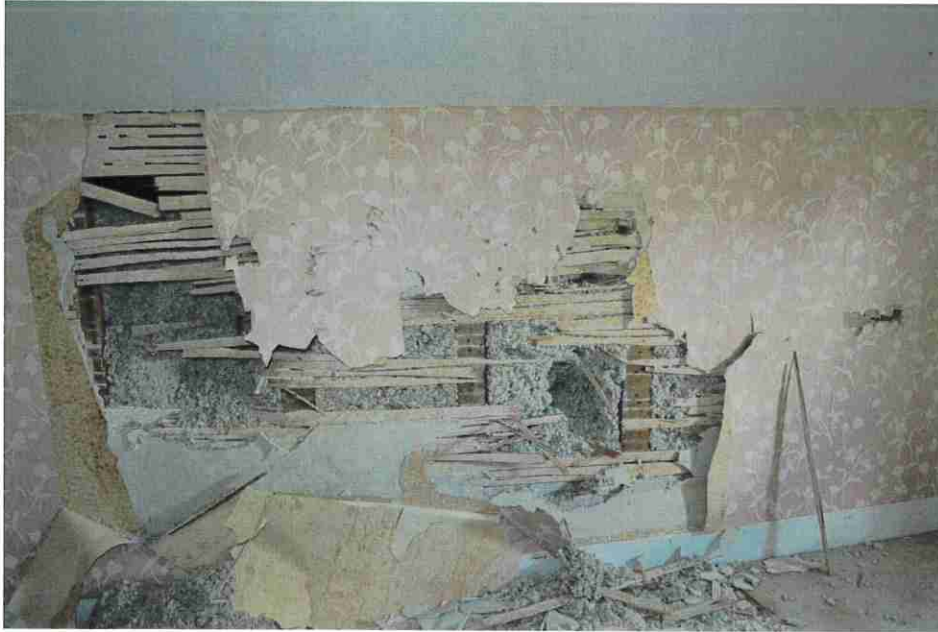
Figure 29: North wall of South east bedroom showing split lath.
