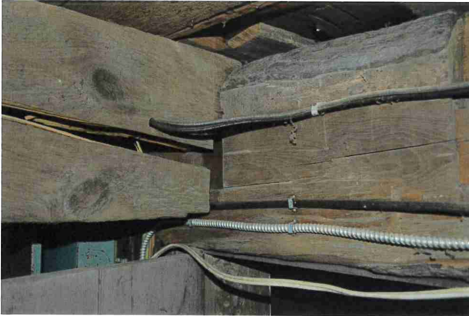
Figure 39: Cellar summer beam on a later brick wall. Note typical joist split because of the insufficient bearing.
