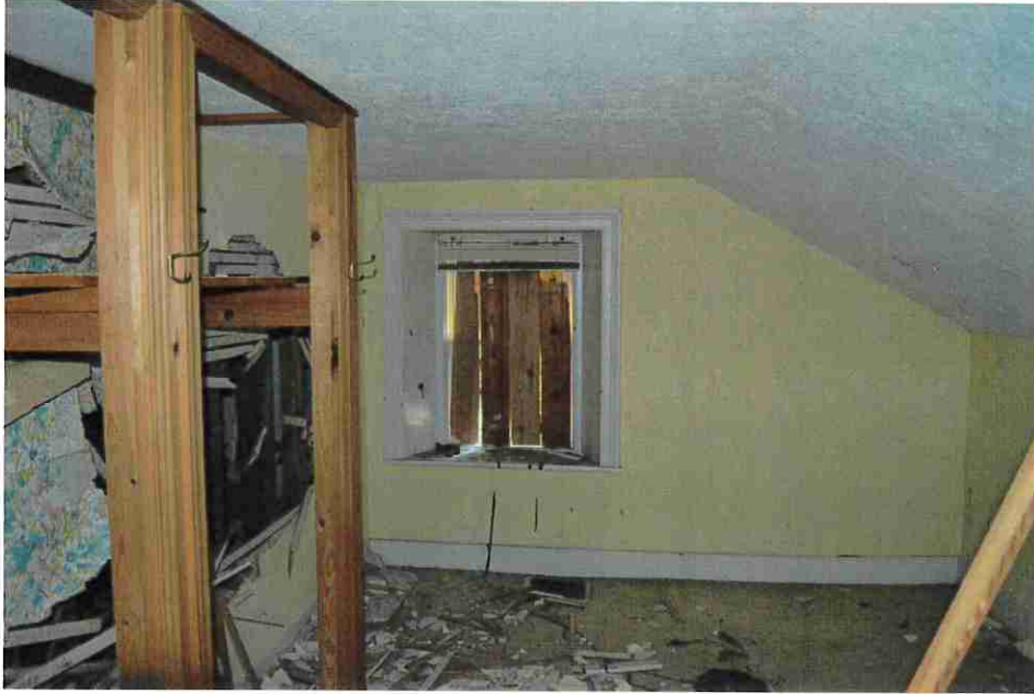
Figure 27: North West Bedroom Note sawn lath. The north two bedrooms were originally combined.
