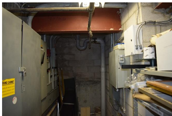
Photo 48: Mechanical room, looking west
