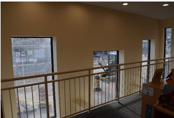
Photo 39: Open space between basement and first storey preserving window openings, looking south
