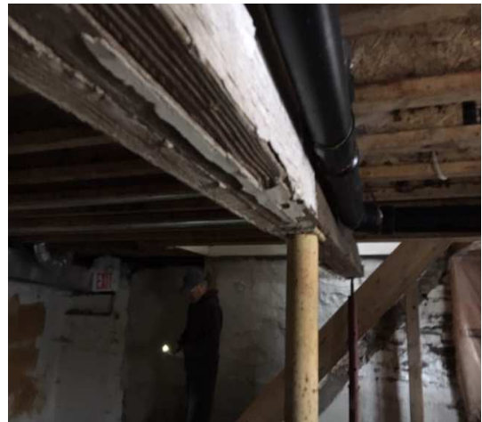
Photo 10 12" deep Main Floor I joists on Wood Bm & Post View Looking West
