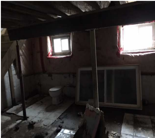
Photo 9 12" Deep Main Floor I joists on Wood Bm & Post View Looking North
