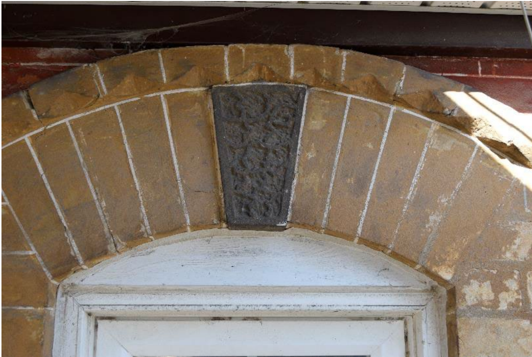
Image 13: Ribbon pointing present in voussoirs
