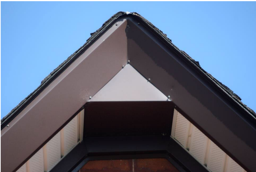
Image 22: Aluminum fascia used to cover suspected attachment point of drop pendant decoration
