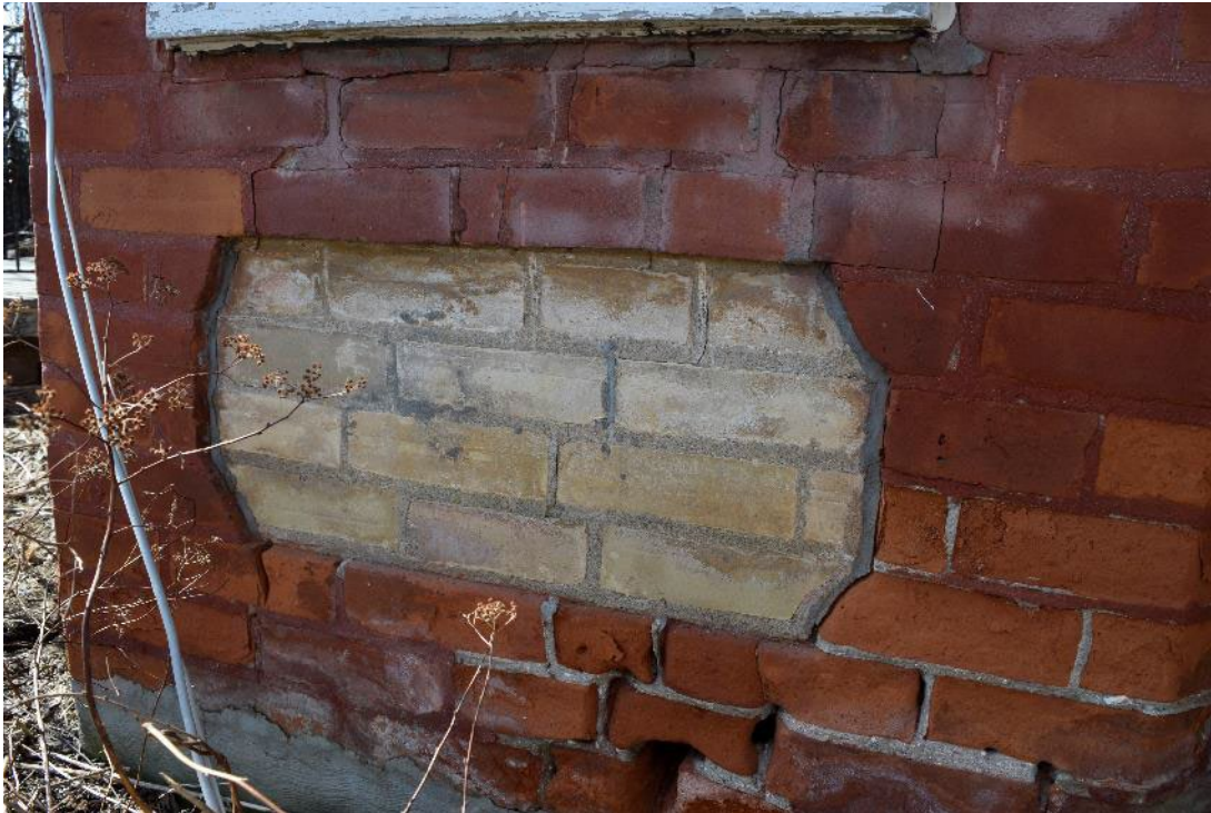
Image 17: Closeup of brick panels located below structural openings on bays, note extensive water damage to brick and mortar
