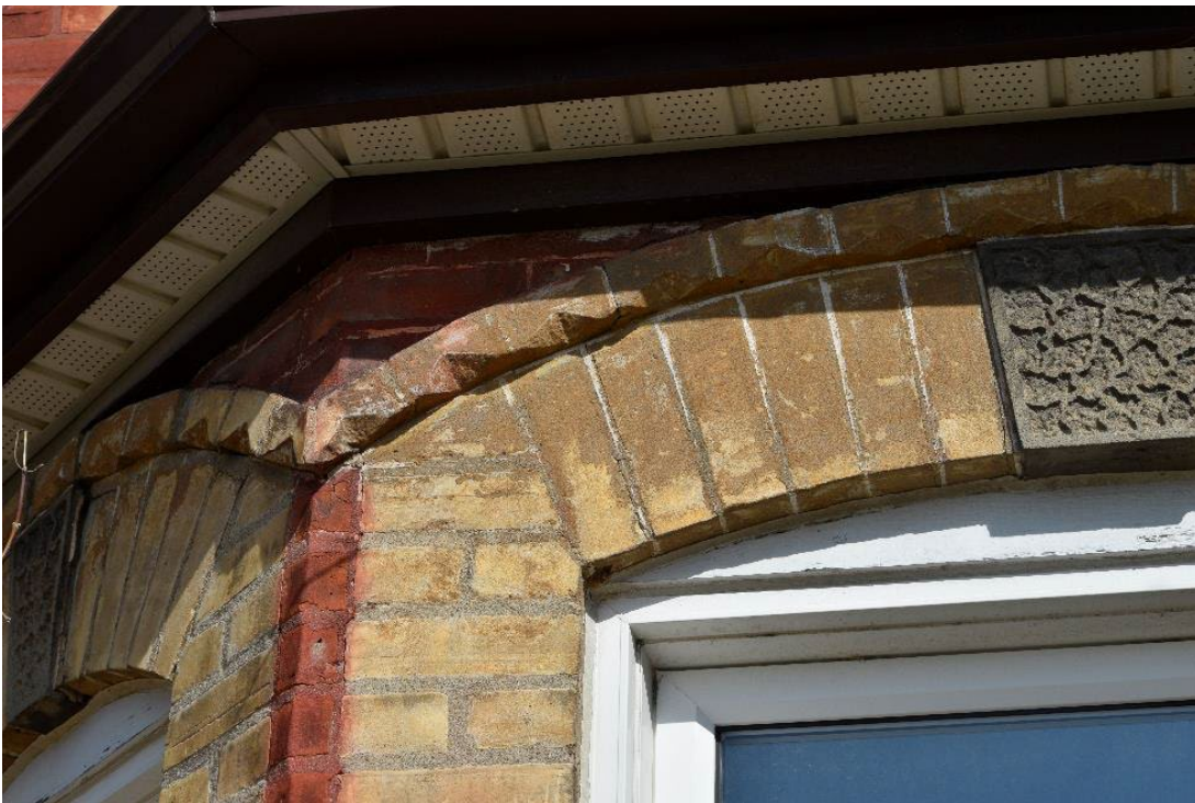
Image 12: Close up of voussoirs with decorative cut buff brick finish as used on east and south face of structure
