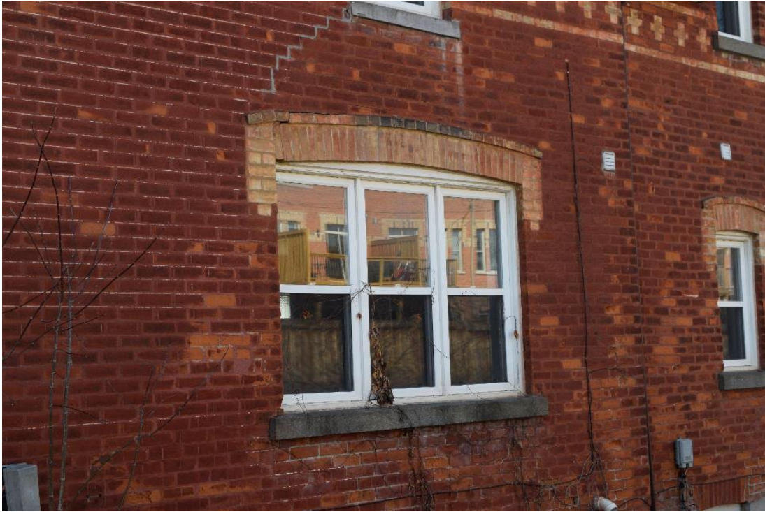
Image 27: Large window on north face of structure, sill has been replaced with cast concrete and voussoir shows signs of deformation
