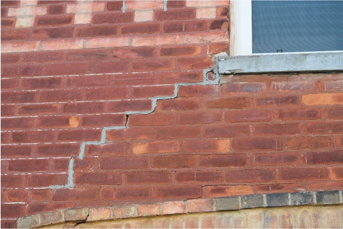
Image 26: Example of cracking in brick veneer
