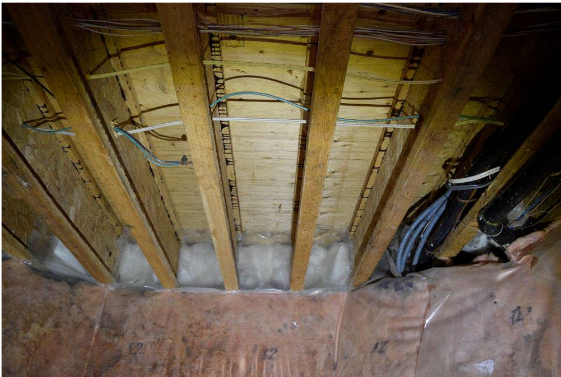
Image 50: I-joists used to replace original floor joists, typical of entire first floor as seen from basement
