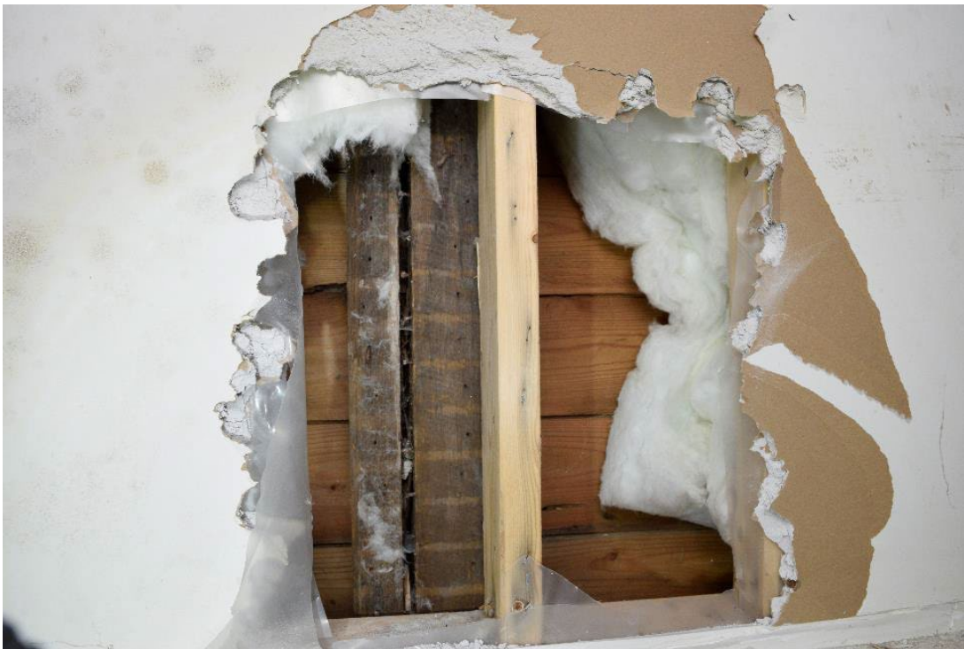
Image 46: Example of original framing with horizontal board sheathing augmented by modern 2x4 framing
