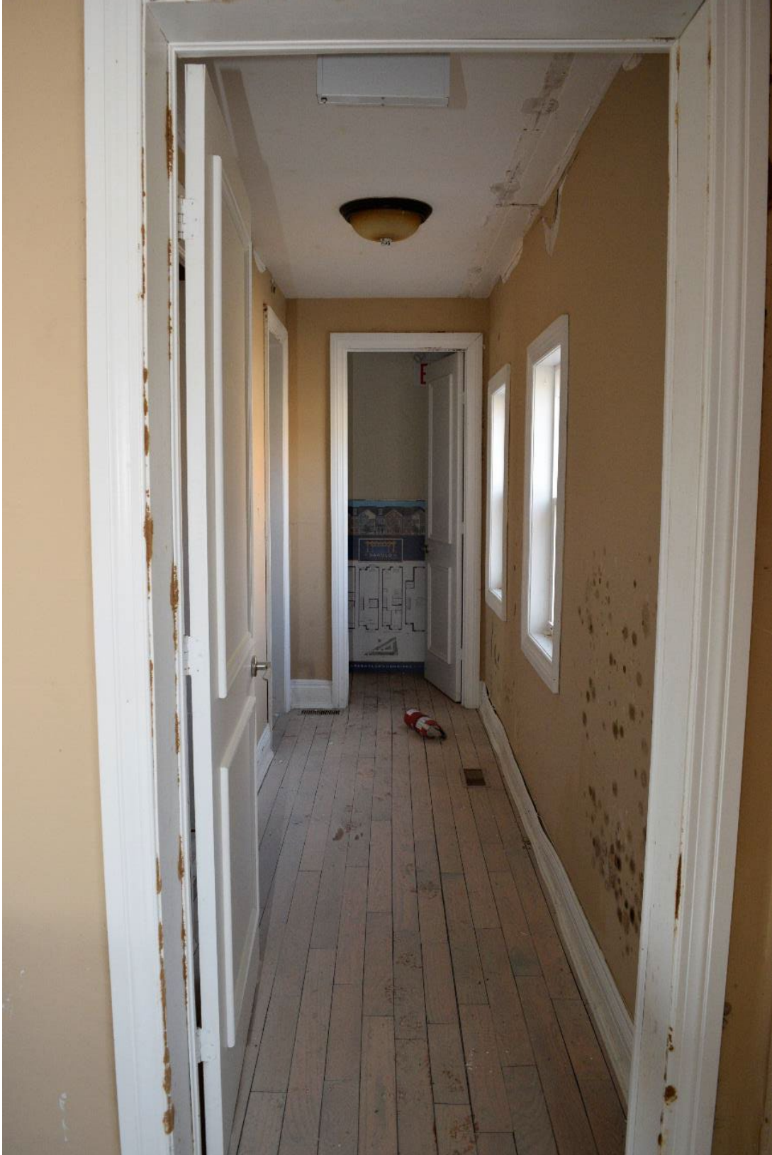
Image 34: Rear hall on first floor, note mould growth and floor damage indicative of extensive water damage, facing west
