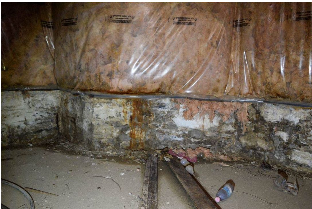
Image 48: Typical example of water damage and mould growth in basement
