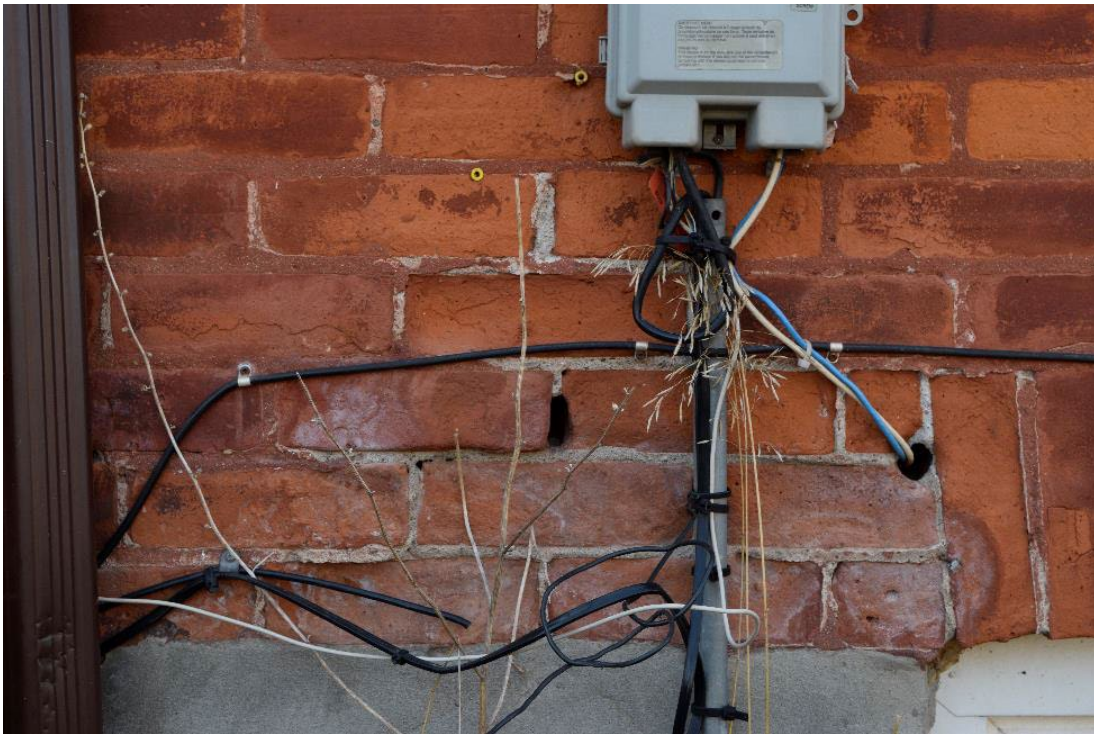
Image 28: Example of typical brick exfoliation resulting from poor water management
