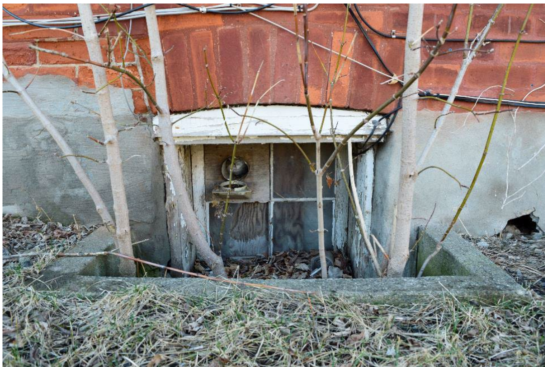
Image 8: Only remaining original wood window, four light awning style in basement window well
