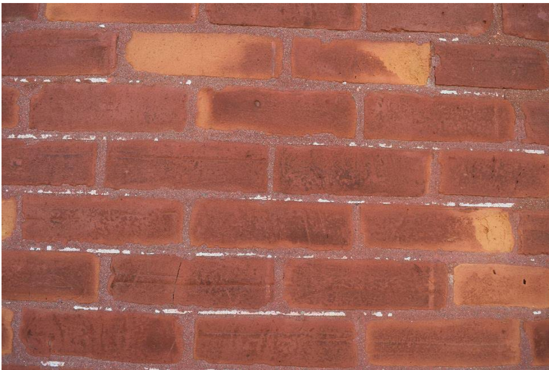
Image 18: Closeup of remaining ribbon pointing in brick façade
