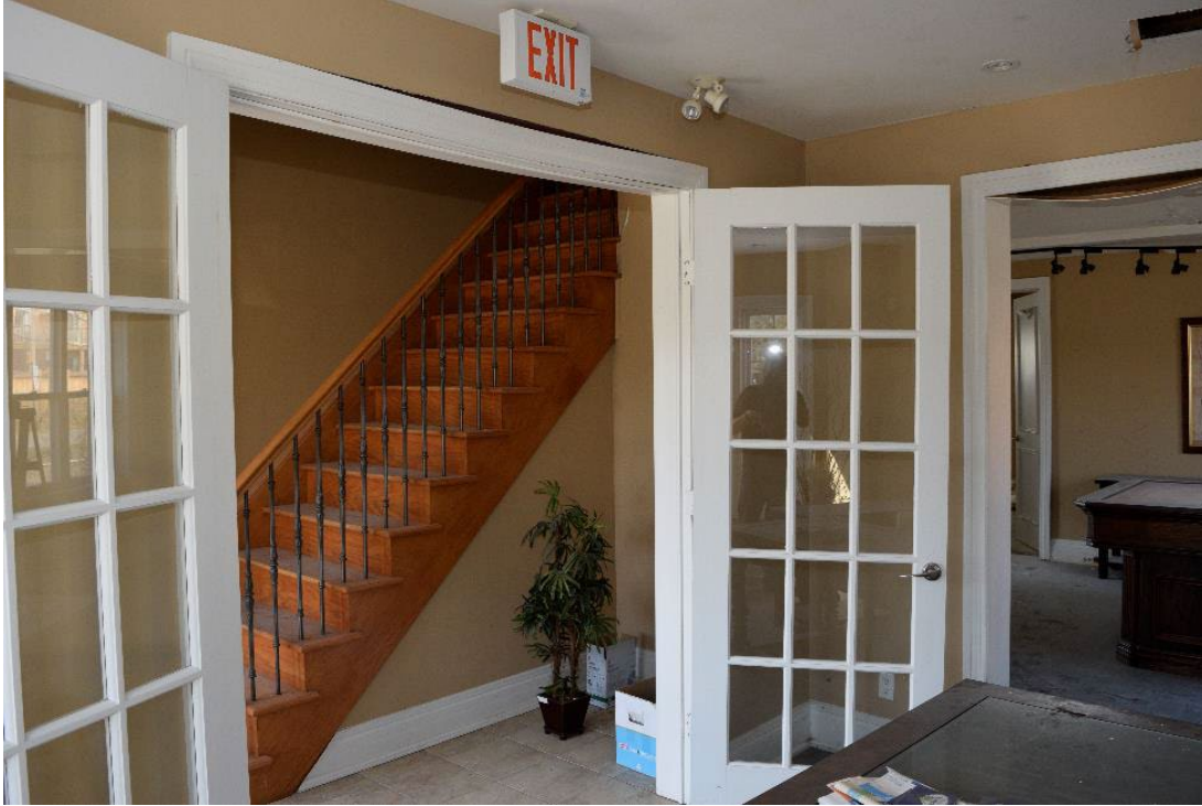
Image 30: Extant stairs, note deformation of trim around door resulting from water infiltration
