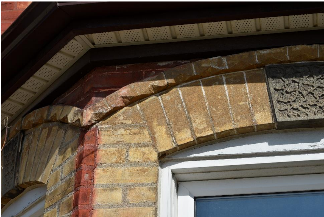
Image 16: Close up of voussoirs with decorative cut buff brick finish as used on east and south face of structure.
