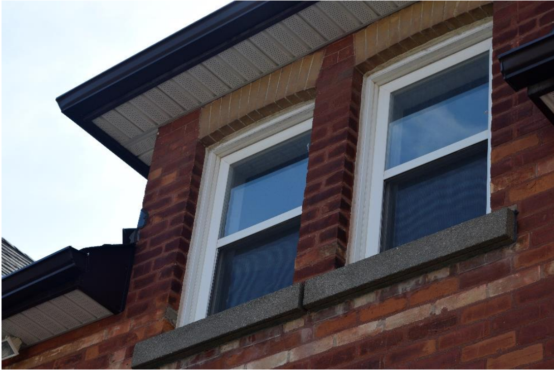
Image 29: Modification to north dormer of structure, sill is cast concrete and brick work does not match with rest of home.
