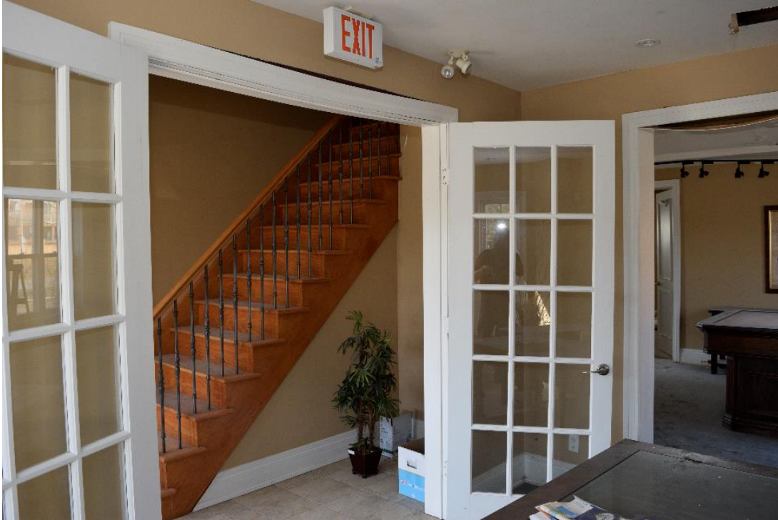
Image 34: Extant stairs. Note deformation of trim around door resulting from water infiltration.
