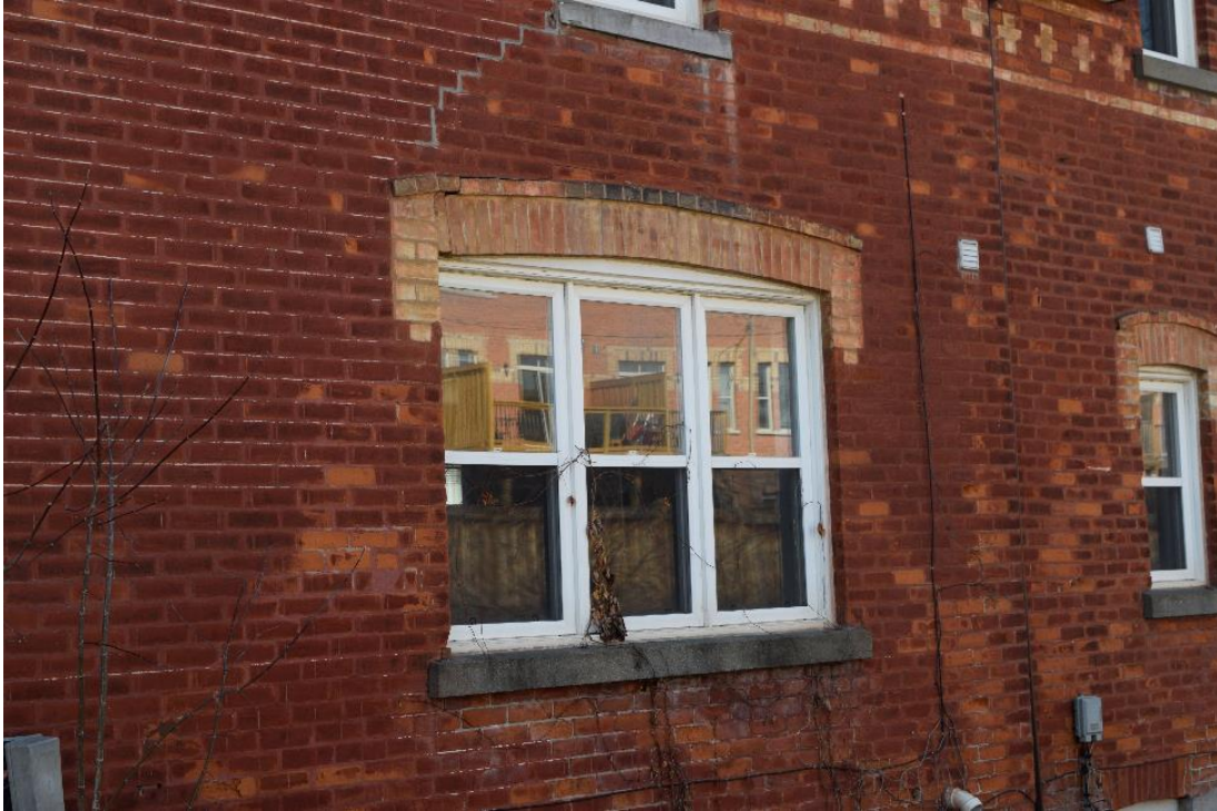
Image 31: Large window on north face of structure, sill has been replaced with cast concrete and voussoir shows signs of deformation.
