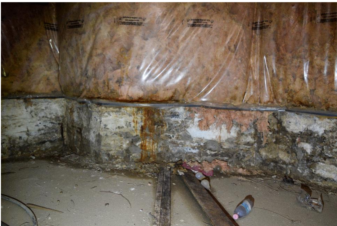
Image 52: Typical example of water damage and mould growth in basement.
