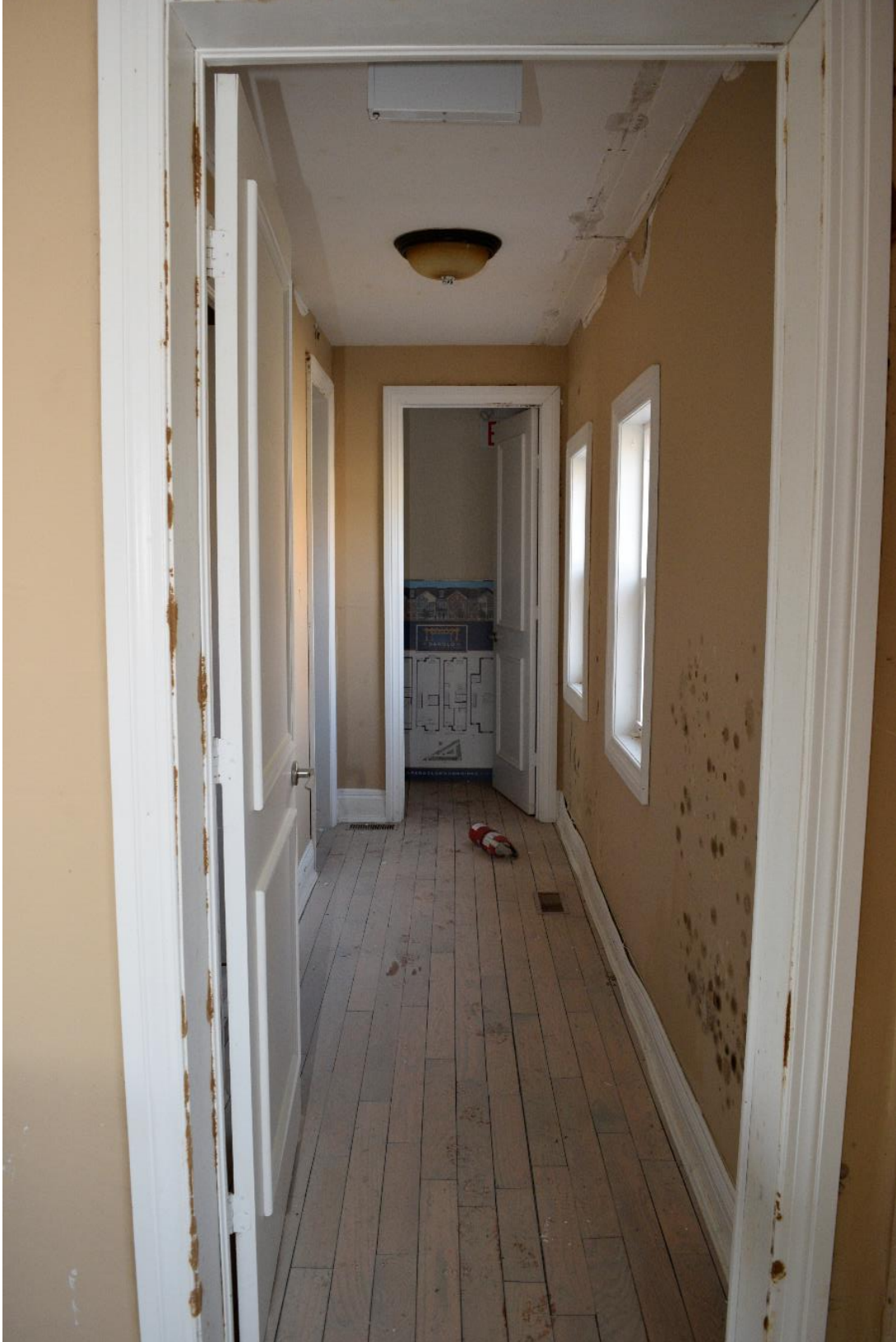
Image 38: Rear hall on first floor, note mould growth and floor damage indicative of extensive water damage, facing west.
