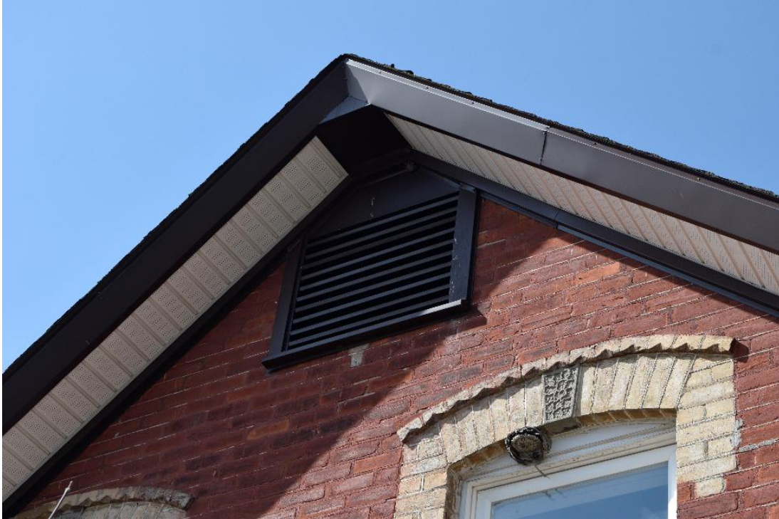
Image 27: Large air vent located in gable end of front façade, note remains of original diamond dichromatic brickwork below grate.
