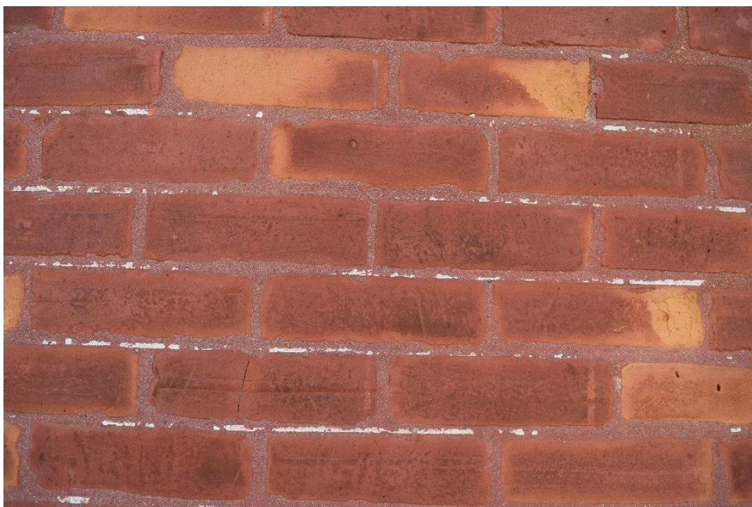
Image 22: Closeup of remaining ribbon pointing in brick façade.
