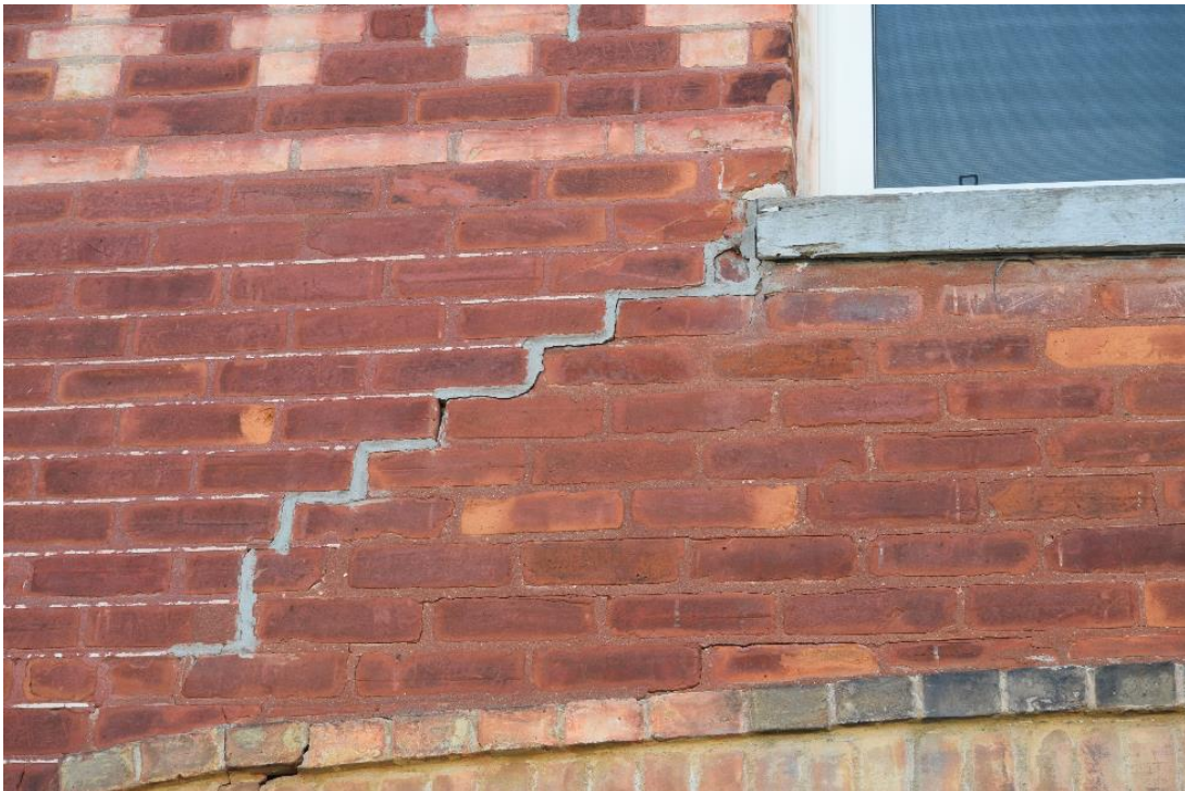
Image 30: Example of cracking in brick veneer.
