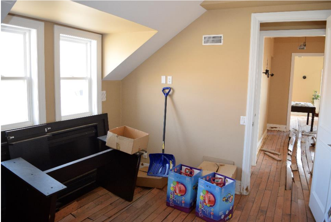
Image 45: Rear room on second floor, facing north. Windows are located in hip dormer depicted in Image 27. Note water damage to flooring.
