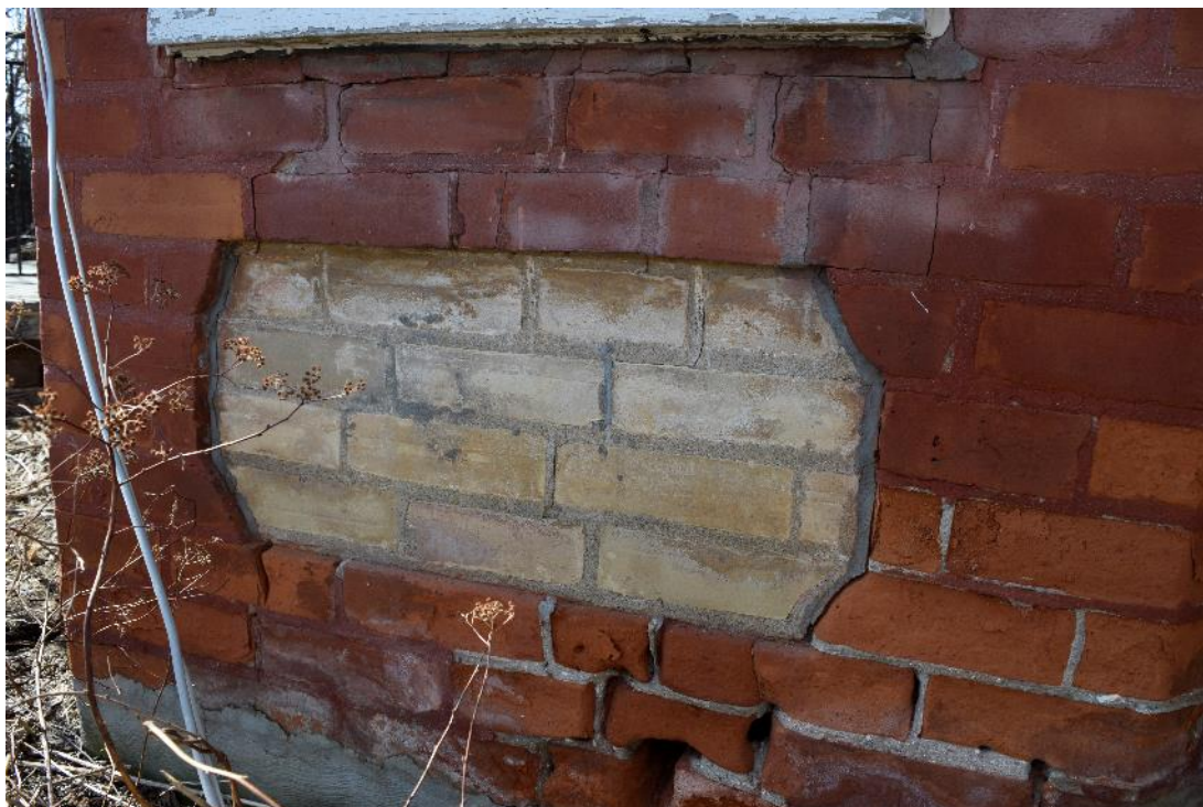
Image 21: Closeup of brick panels located below structural openings on bays. Note extensive water damage to brick and mortar at foundation.
