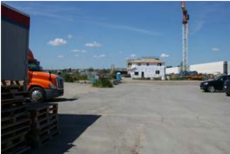
14. View towards the rear (west) half of the lot, with temporary construction training structures visible beyond a large asphalt parking pad.
