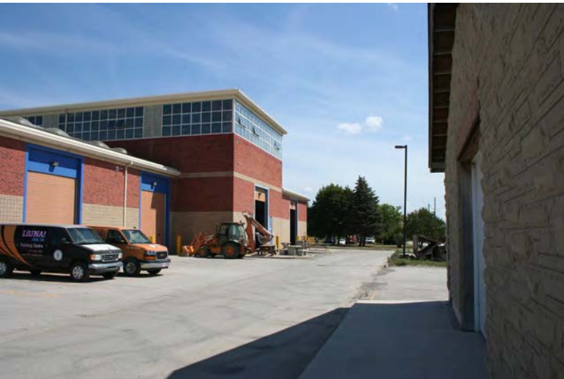
41. View along the south laneway towards the eastern frontage of the lot on Huntington Street. Note that the structure on the right will be demolished to accommodate the new structure on the same site with a larger footprint, and despite this clear view of the laneway, the BHR is not yet visible.
