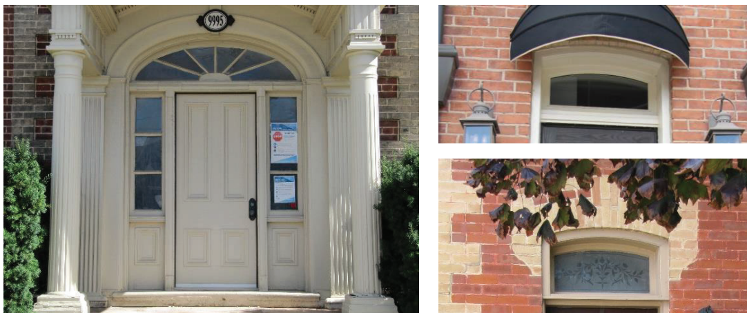
Photo 4-8: Examples in HCD of original door sidelights, fanlight, mouldings, and segmental transoms
