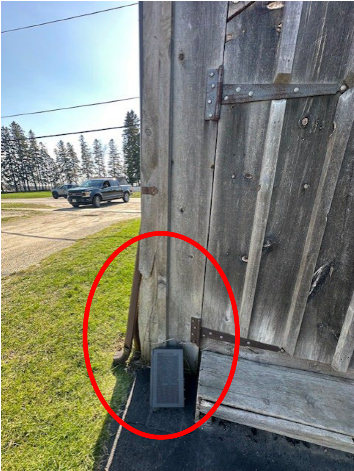
Structural damages on the southeast side of the barn
