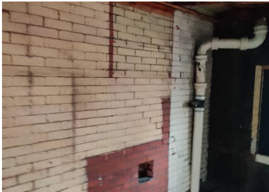
Figure 41. Settlement cracking second floor rear wall.
