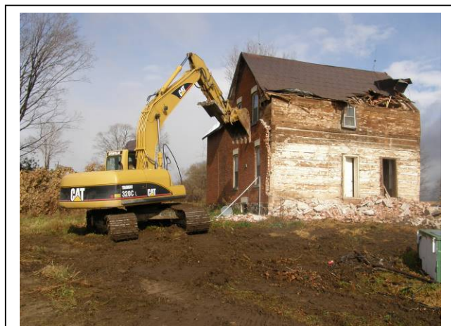
Figure 45. Stripping brick veneer from another log house, this one in Stroud. It's fast work for a skilled operator. Photo by Vic Snow.
