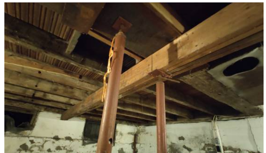
Figure 45. The ground floor framing, including the summer beam, has required some additional support. Unknown if this is related to the steel beam installed above.
