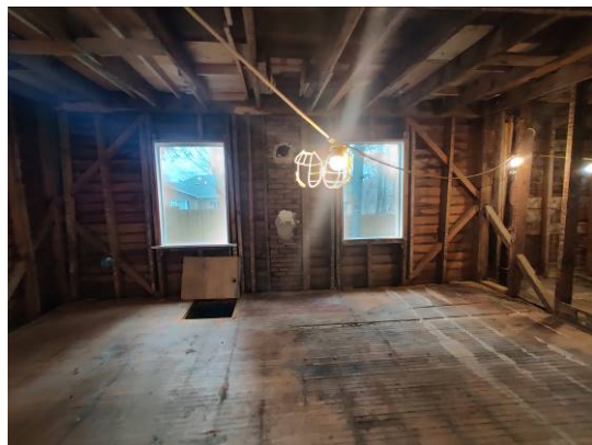
Figure 25. Northeast corner, with kitchen tail to the right. The mortised bracing of the corner post is very evident here.
