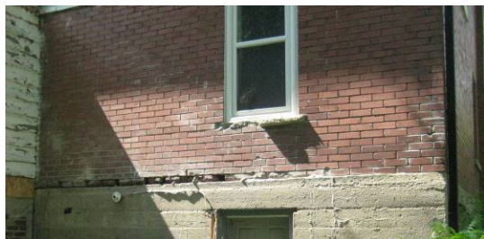
Figure 36. This sill on the rear wall has almost completely fallen apart. The bottom course of brick is crumbling, for reasons unknown, and the mortar has eroded in the lower right corner.
