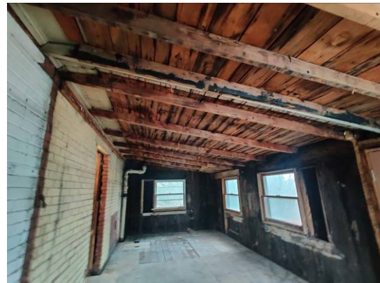
Figure 20. Standing in the east room on the second floor, looking north. Because the brick has already been installed on the main house, we know that this room is a later addition.
