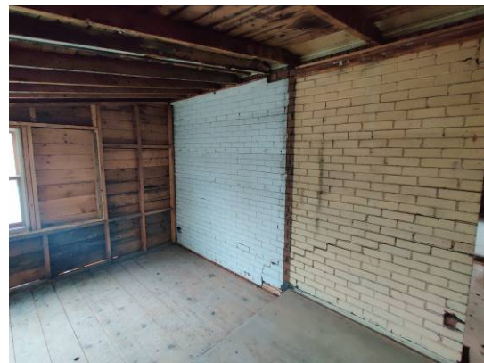
Figure 40. Settlement cracking, second floor rear wall.
