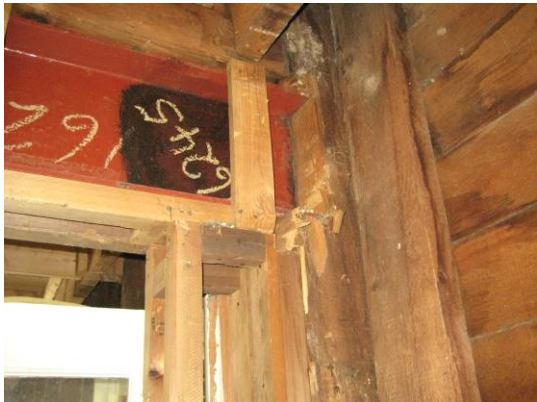
Figure 42. At some point a bearing wall on the ground floor was removed and replaced with a steel beam. It rests on a notch in the original framing and this timber salad. In my professional opinion, this is not proper bearing. My photo.
