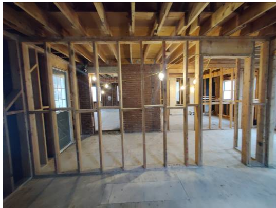
Figure 18 Near the south end of the south addition, looking north. The brick panel is the southeast corner of the main house.
