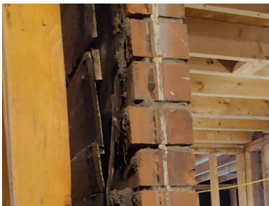
Figure 43. This was once an exterior wall: from left (inside) to right (outside)—stud, clapboard, roofing felt, air gap, brick. There might be some kind of ties between the brick but we haven't found any.
