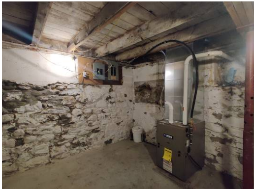
Figure 12 looking to the southeast corner. Note lower foundation of fieldstone & concrete above.
