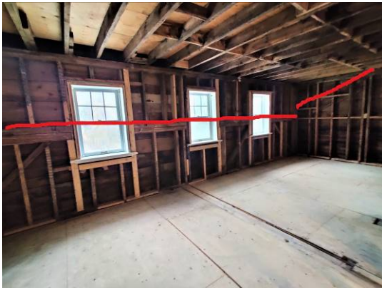
Figure 30. The red line on the left follows the top of the original header beam. It has been cut to fit the windows. The red line to the right follows the line of the original gable header. Everything above these lines was added—most likely at the time of the brick veneer installation.
