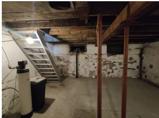
Figure 11. The basement extends under the original house, and additions are unexcavated. This view is from the middle of the main body of the house to the northeast corner. A steel post and timber beam have been installed to support the original heavy timber summer beam, which is also supported by a second steel post.
