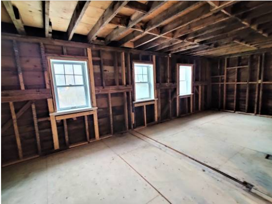
Figure 29. Looking to the northwest corner upstairs: another surprise. The house was once a half-storey smaller.
