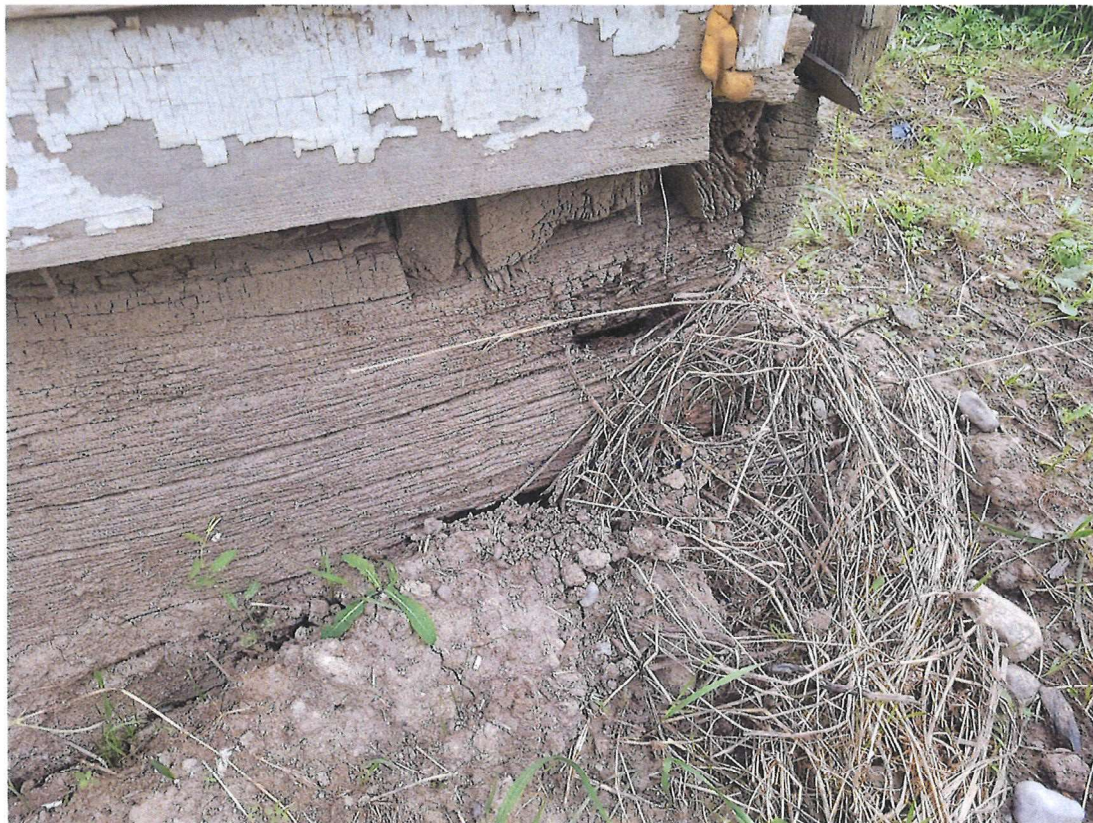
Photo 2 - Typical view of exterior showing deterioration of exterior portions of logs
