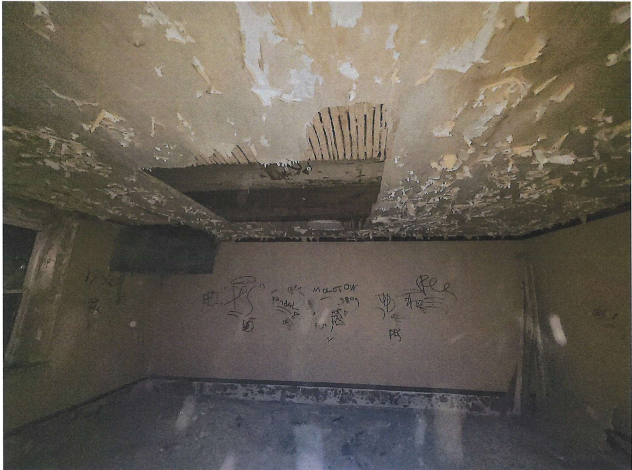
Photo 3 - Typical view of interior showing deteriorated finishes
