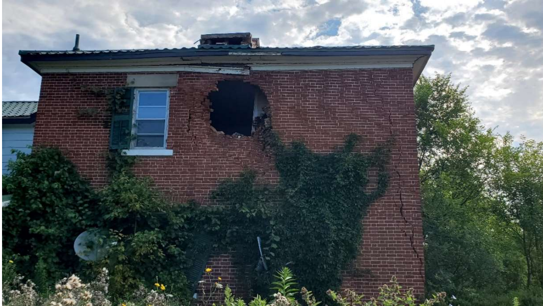
Pic. 3: Westview showing Cracks on the Masonry Wall, Part Caved In and Broken Chimney
