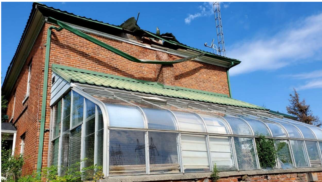
Pic. 7: Eastside View of the House showing Damaged Roof at Broken Chimney and Greenhouse Addition
