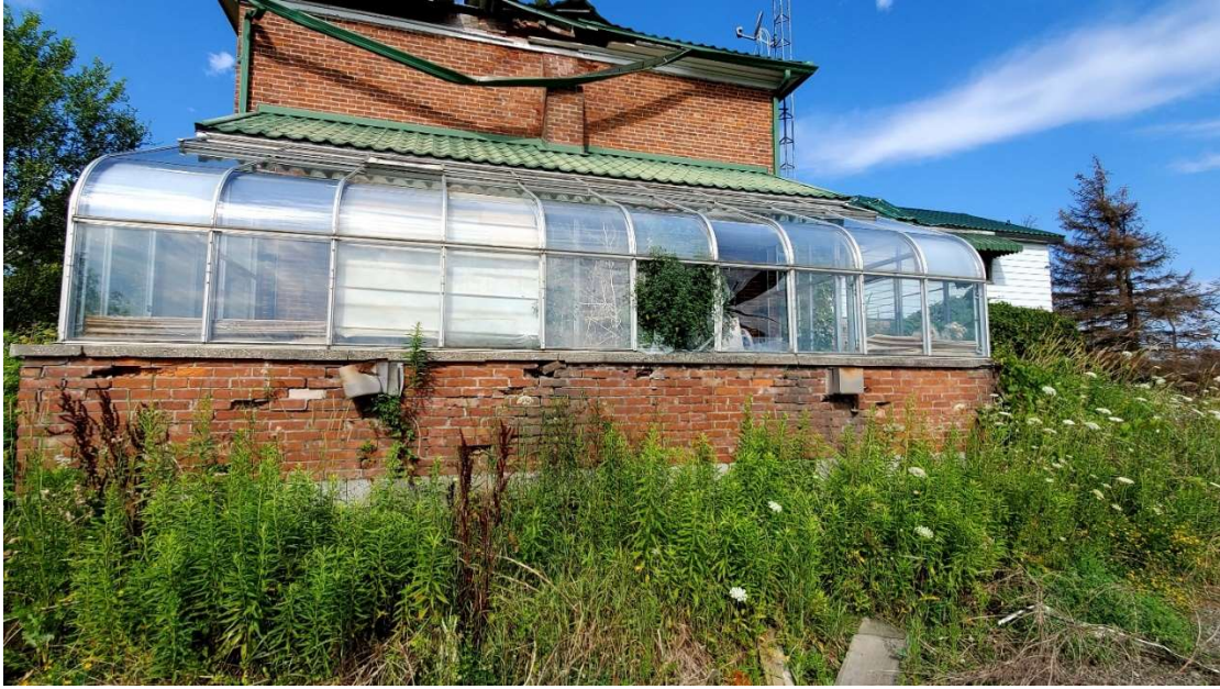
Pic. 8: Eastview showing disintegrated Masonry Wall, Vegetation growth in the Greenhouse with Broken Panes
