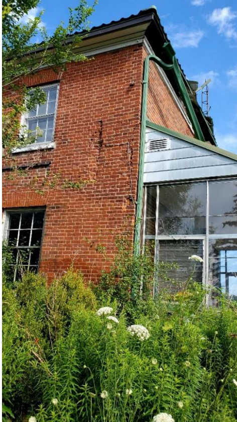
Pic. 6: Cracks and Damage on the Southside Masonry Wall of the House
