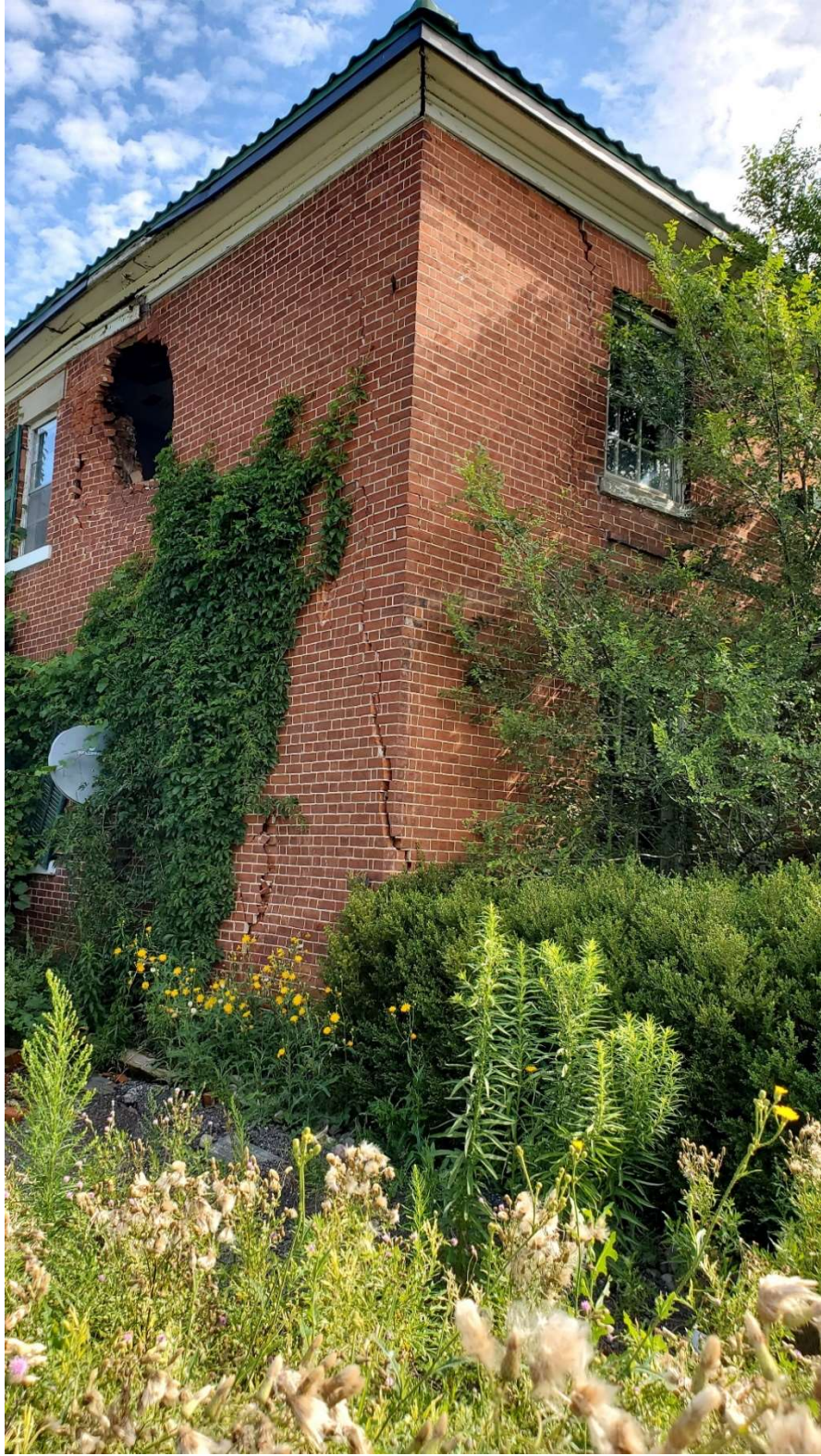
Pic. 5: Southwest view of the House-Cracks and Damage in the Load-bearing Masonry Wall
