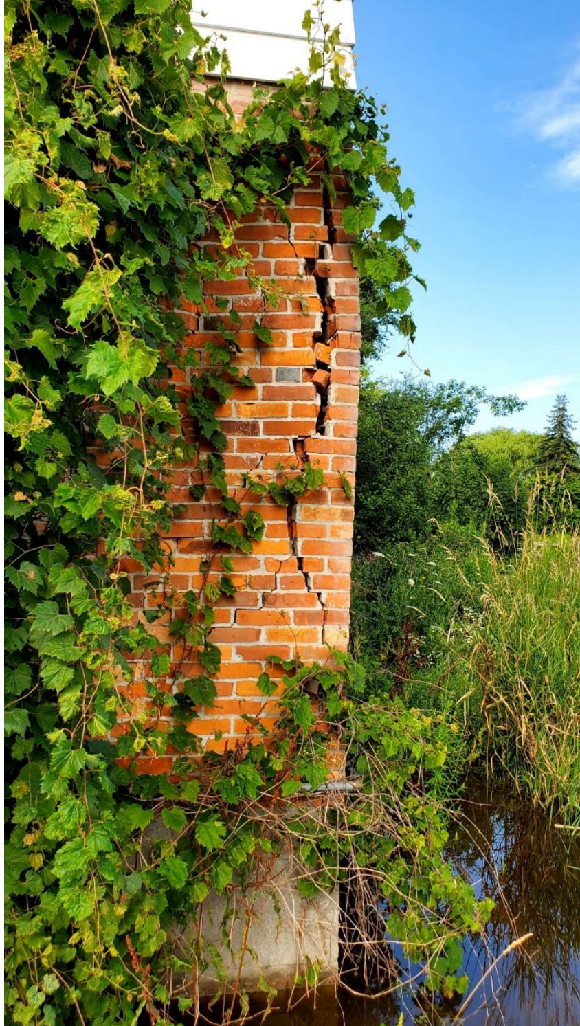
Pic. 10: Wide and Long Vertical Crack on the Northside House Addition and Water Pool Outside
